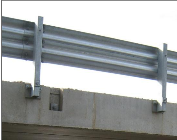
e. Guardrail system
