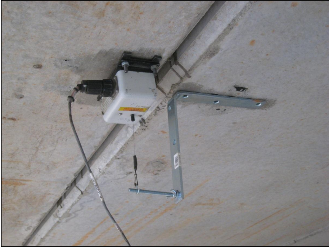
Figure 3.2. Relative displacement transducer between DBs 5 and 6
