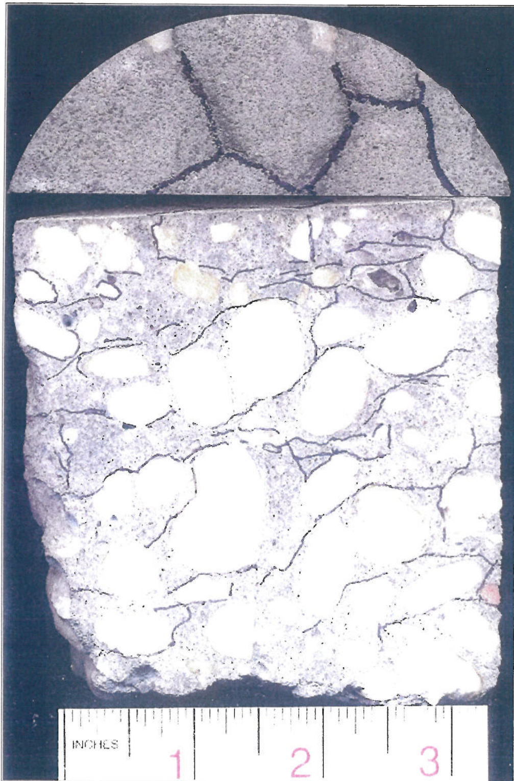
Figure 5: Plan view (top photo) and corresponding cross sectional view (bottom photo) of the core showing the pattern of map cracking at the surface and subparallel cracks in the body of the concrete transecting and circumscribing the aggregate particles.
