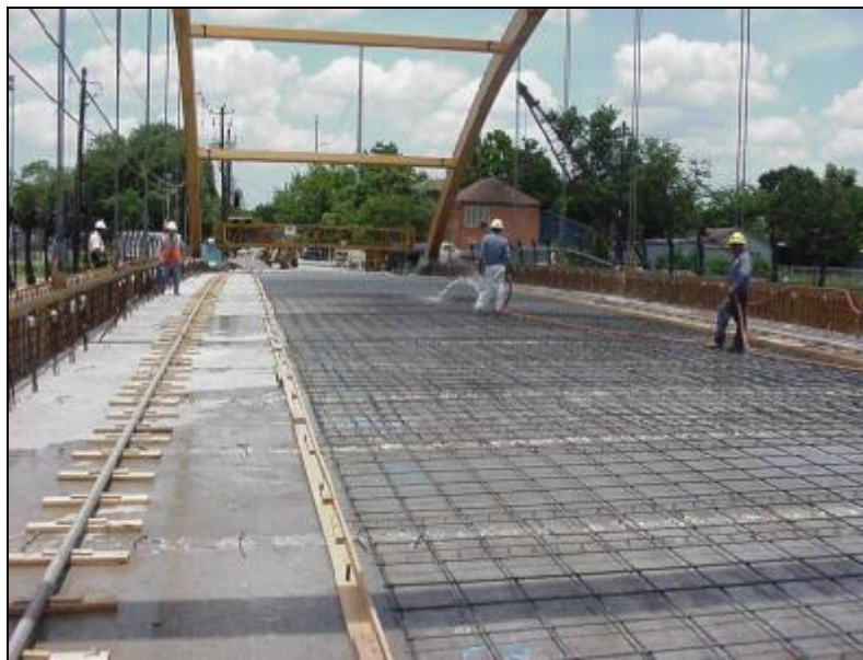
Figure A.2.4.11-8 Reinforcement of the cast-in-place topping of the arch tied bridge
