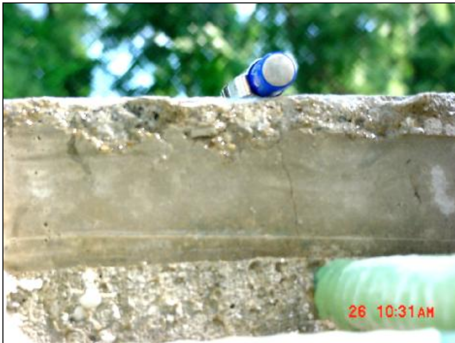
Figure A.2.4.9-7 Side view of the panel showing the top surface crack penetrating the top surface to the reinforcement level
