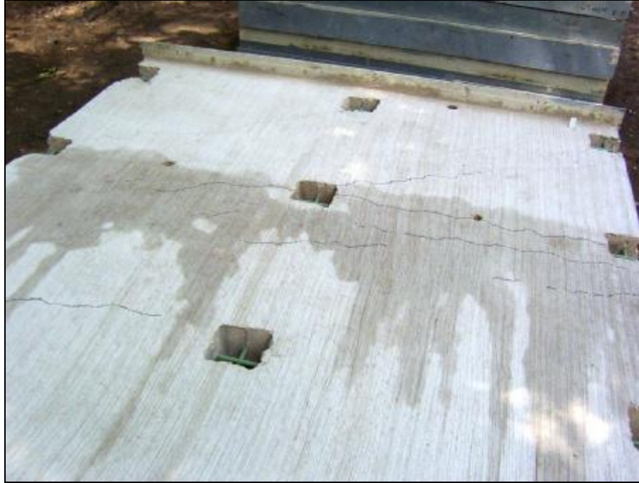
Figure A.2.4.9-6 Top view of the panel showing the top surface cracks
