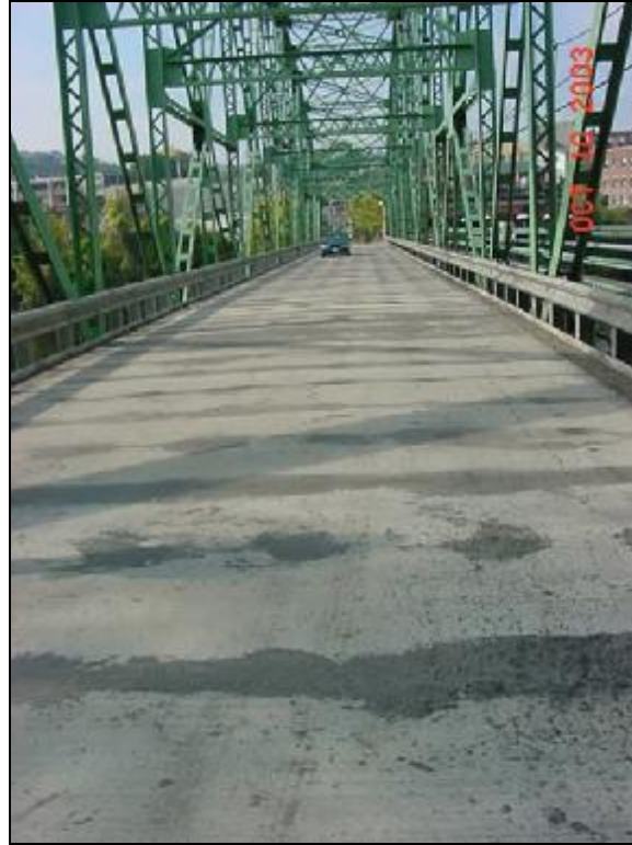
Figure A.2.4.9-8 General view of the bridge shortly after it was open to traffic
