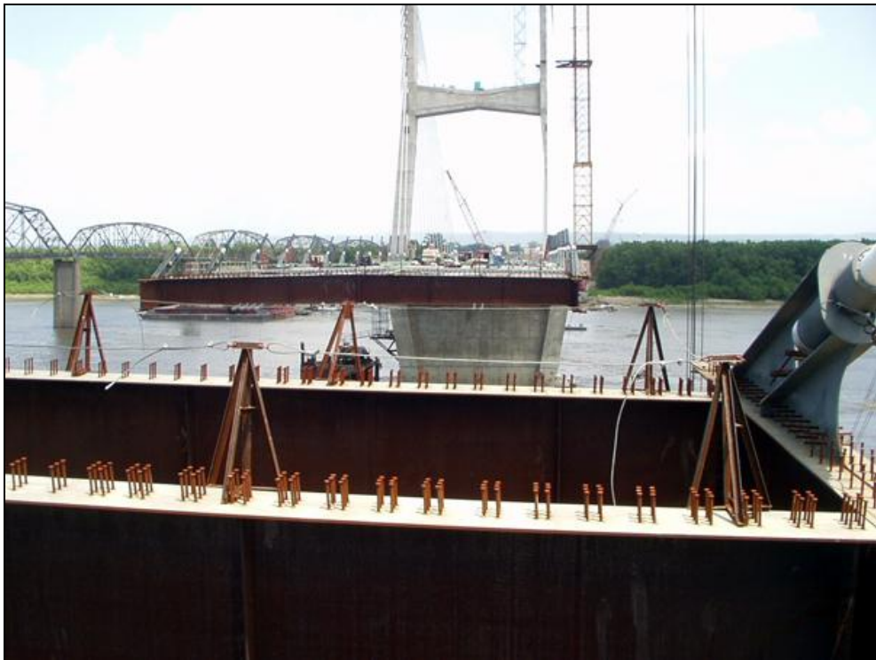
Figure A.2.4.6-4 Steel studs welded to the top flange of the girders and floor beams
