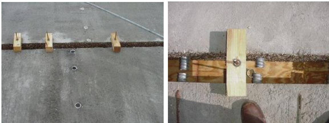
Figure A.3.2.2-2 Wood forming of the panel-to-panel joint used in the Arch Tied Bridges, Texas
