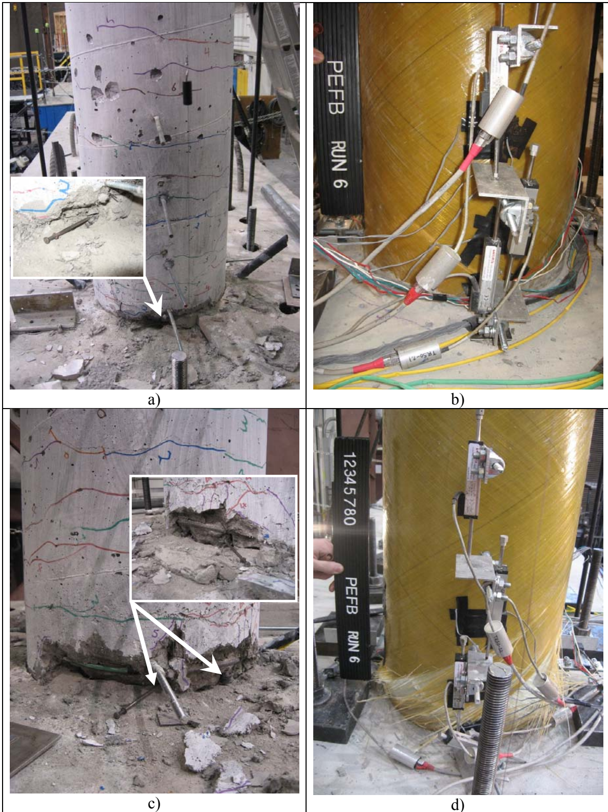
Fig. 4-12. Apparent Damage at 10% Drift for a) RC-ECC, North, b) FRP, North, c) RC-ECC, South, d) FRP, South
