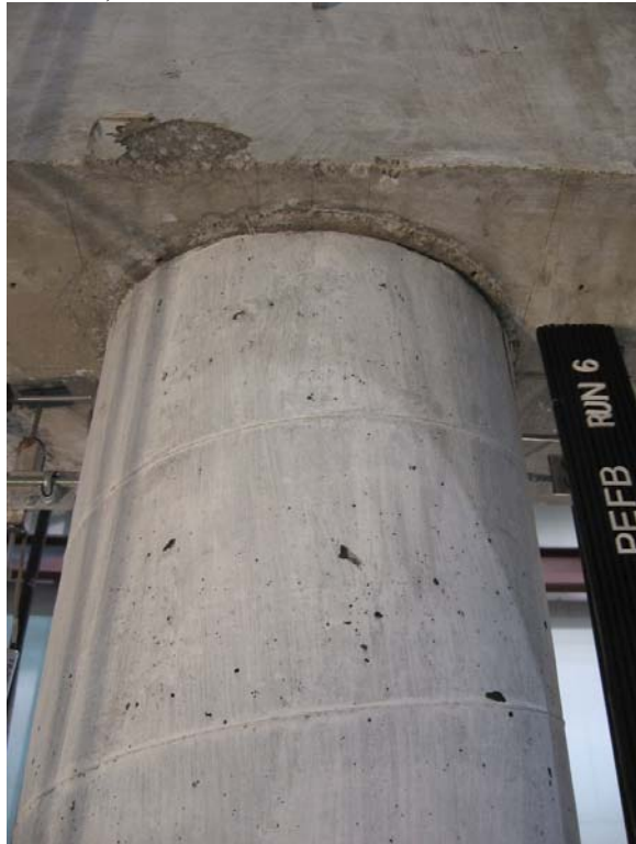
d) RC-ECC Column, West, Run-6
