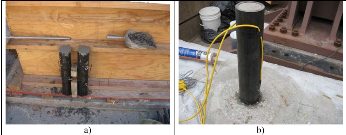
Fig. 2-68. Steel Pipe-Pin, a) Filled with Concrete, b) Sat on the Cap Beam
