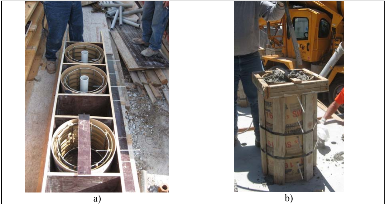
Fig. 2-39. a) Typical Segment Column Cages, b) Constructing the Second Segment with Match Cast Method
