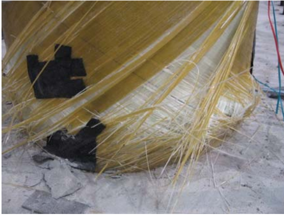
a) FRP Rupture, South, Run 6
