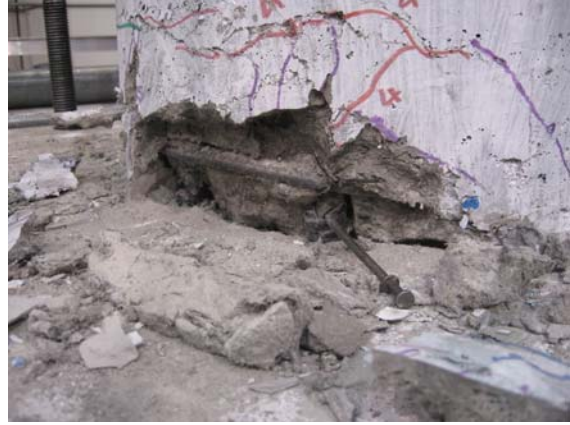
b) RC-ECC Column, South, Run-6
