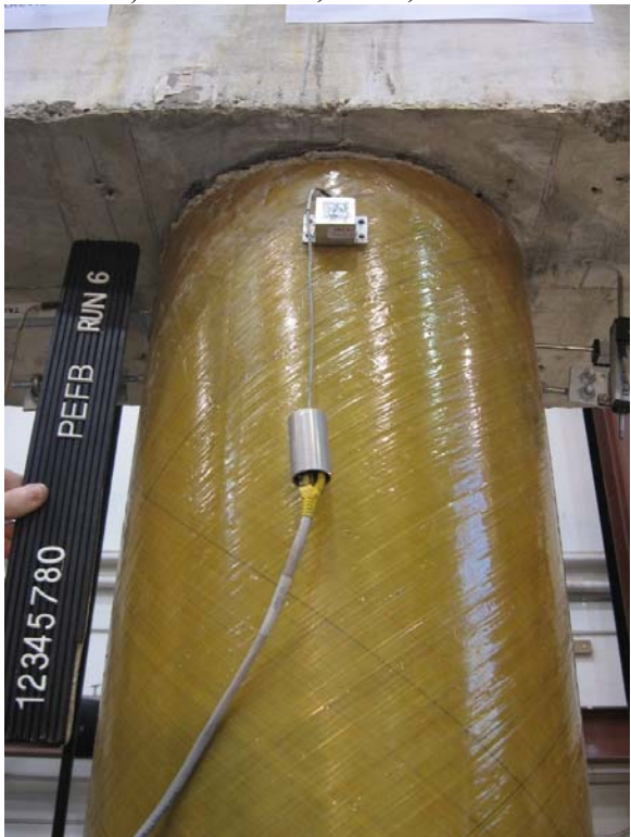
c) FRP Column, East, Run-6
