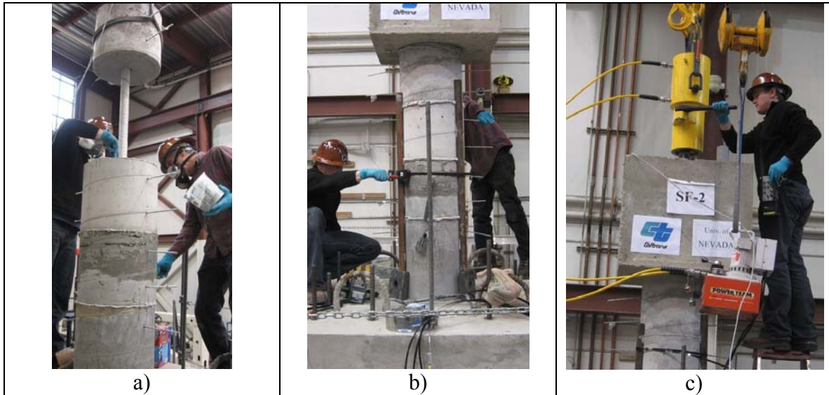
Fig. 2-9. Columns Assembly, a) Setting the Segments, b) Adjusting the Segments, c) Post-Tensioning
