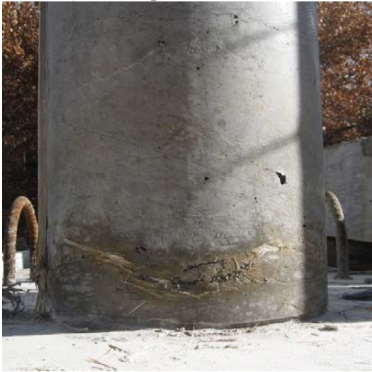
c) Horizontal Crack, South, Run 6
