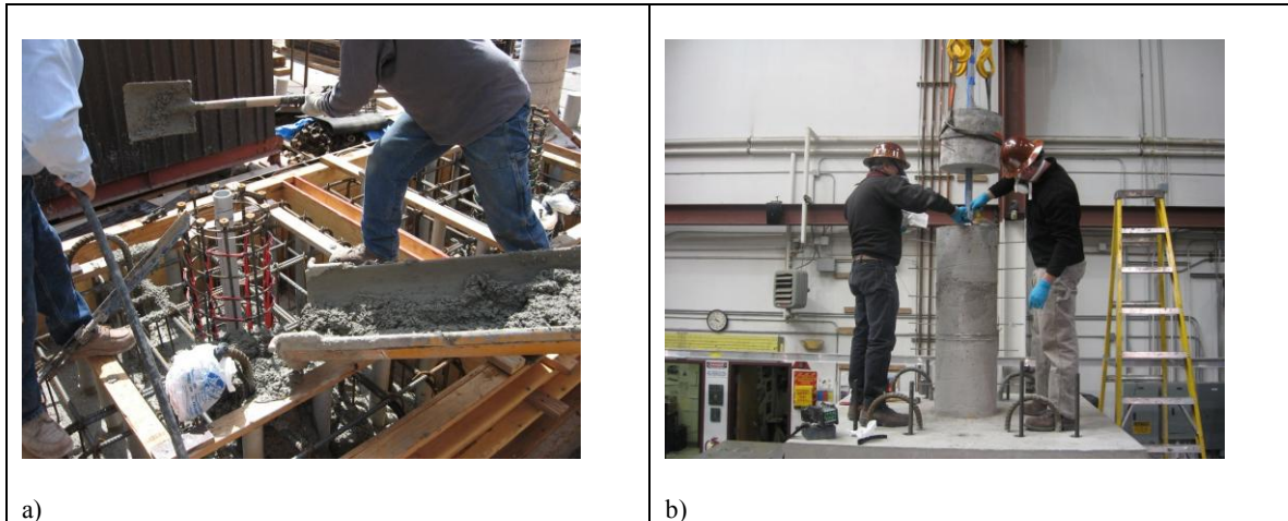
Fig. 4- Footing and the Base Segment steel Cages, b) Assembling Process in Segmental Columns
