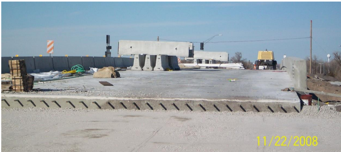
Figure 2.4: I-80 Hershey Interchange project in North Platte, NE after stacking barriers at the mid-span of second phase.
