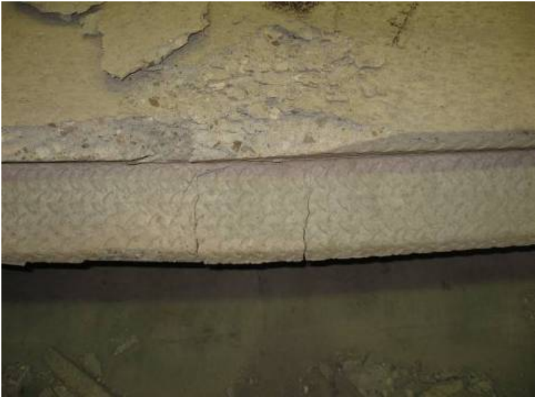
b) Flexure cracks
