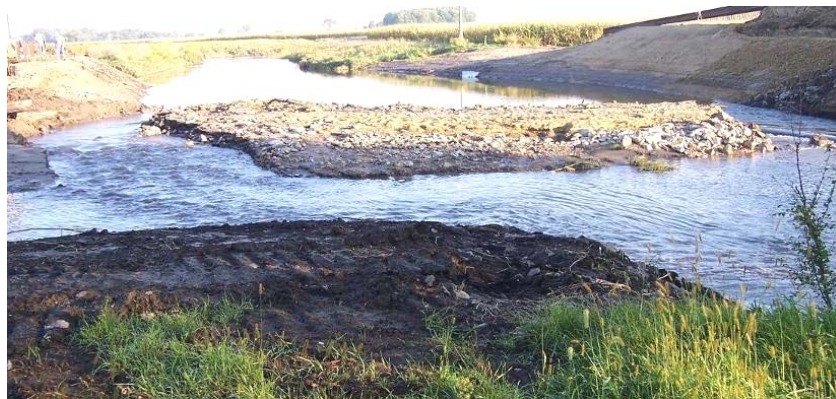
Figure 106. Washed out access road, September 15
