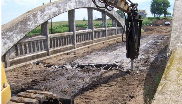
Figure 102. Breaking apart the Marsh Arch bridge deck with a back hoe, July 24
