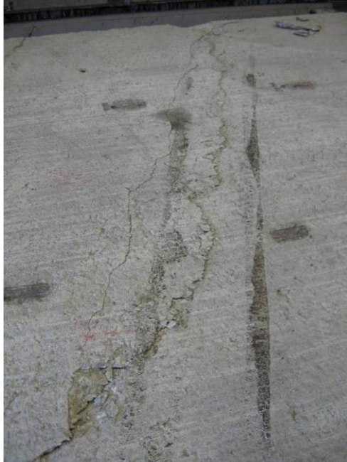
Figure 3.32. Flexural cracking in deck panel due to applied line load
