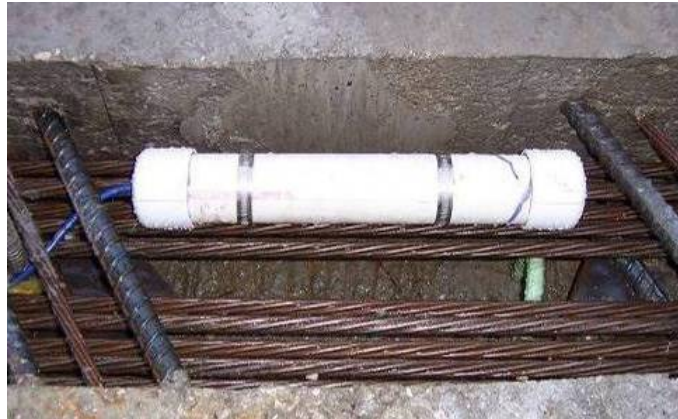
Figure 88. Vibrating wire gage with PVC pipe cover
