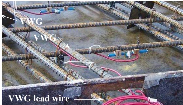
Figure 81. Deck panel vibrating wire gages
