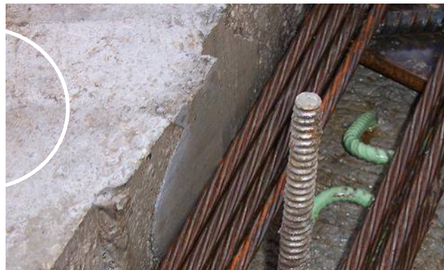
Figure 86. Concrete obstruction in Channel 1
