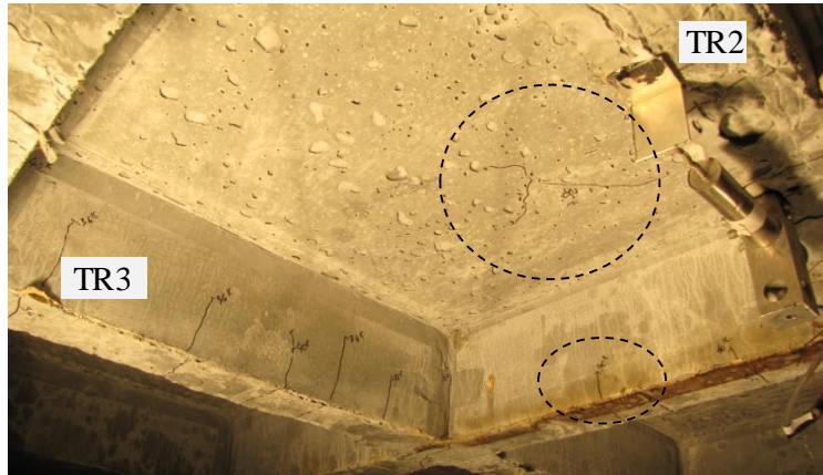
a) Cracking on the bottom surface of the slab and on a longitudinal rib
