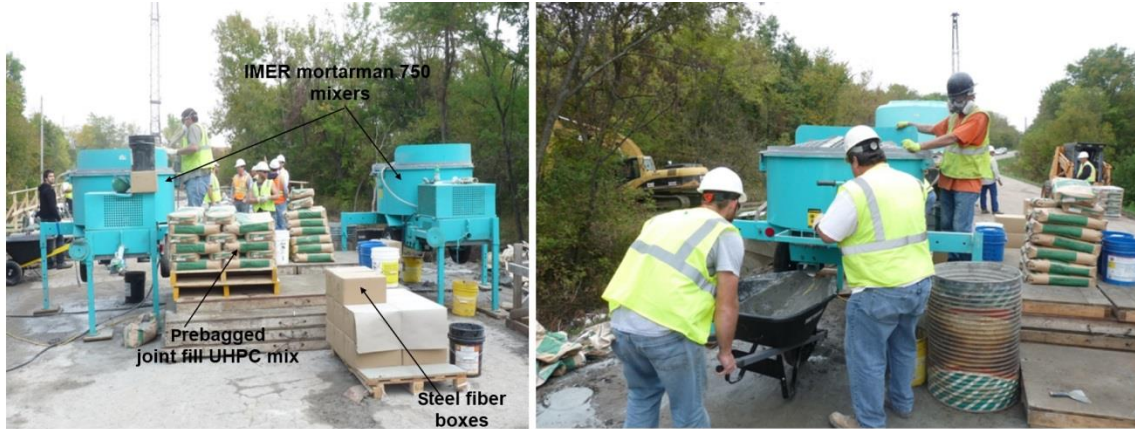
Figure 3.8. Batching of UHPC joint fill using IMER Mortarman 750 mixers at the bridge site
