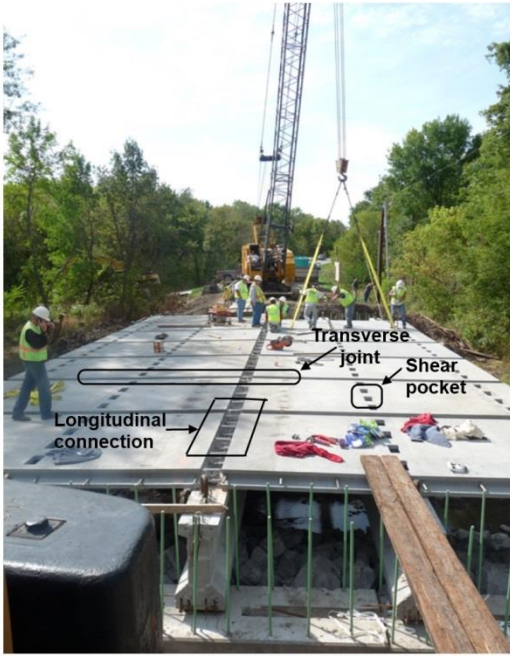
a) Wapello County bridge with UHPC waffle deck panels
