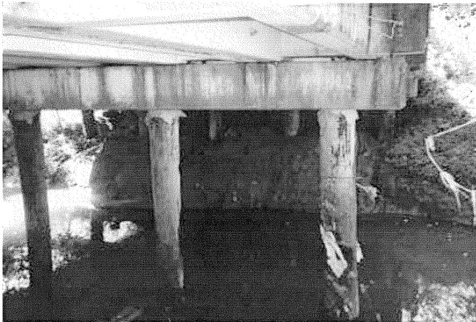
Figure 7 Priority #2, Clinton Tinnon Road over Straight Fence Creek, bridge supports
