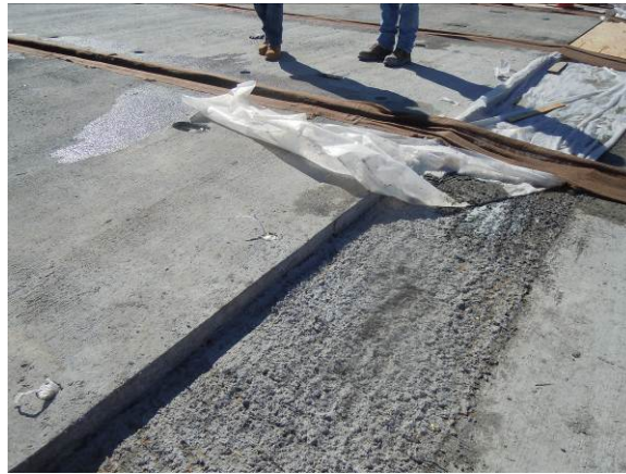
Figure 19. Step resulting from NEXT beam camber.
