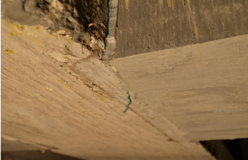
Figure 3.8-15 Bottom view of bridge model showing development of cracks at diaphragm
