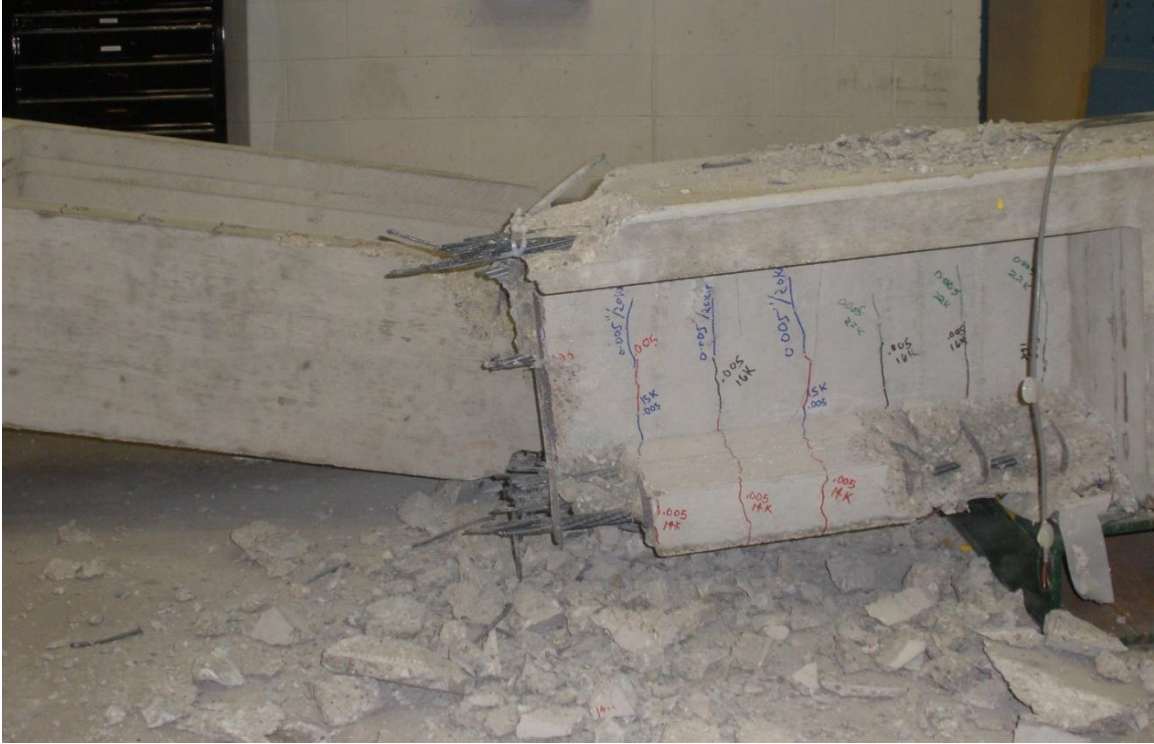
Figure 3.3-2 Balanced failure resulting in complete separation of Beam C-C-F-B
