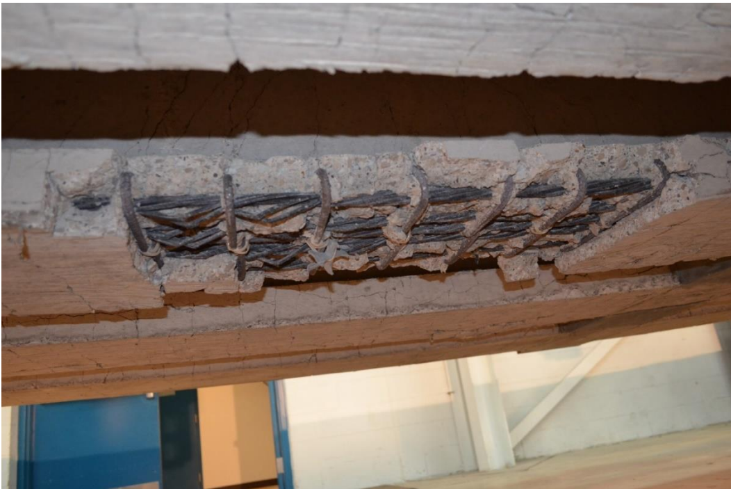
Figure 3.8-28 Spalling of concrete from bottom of loaded intermediate beam at failure
