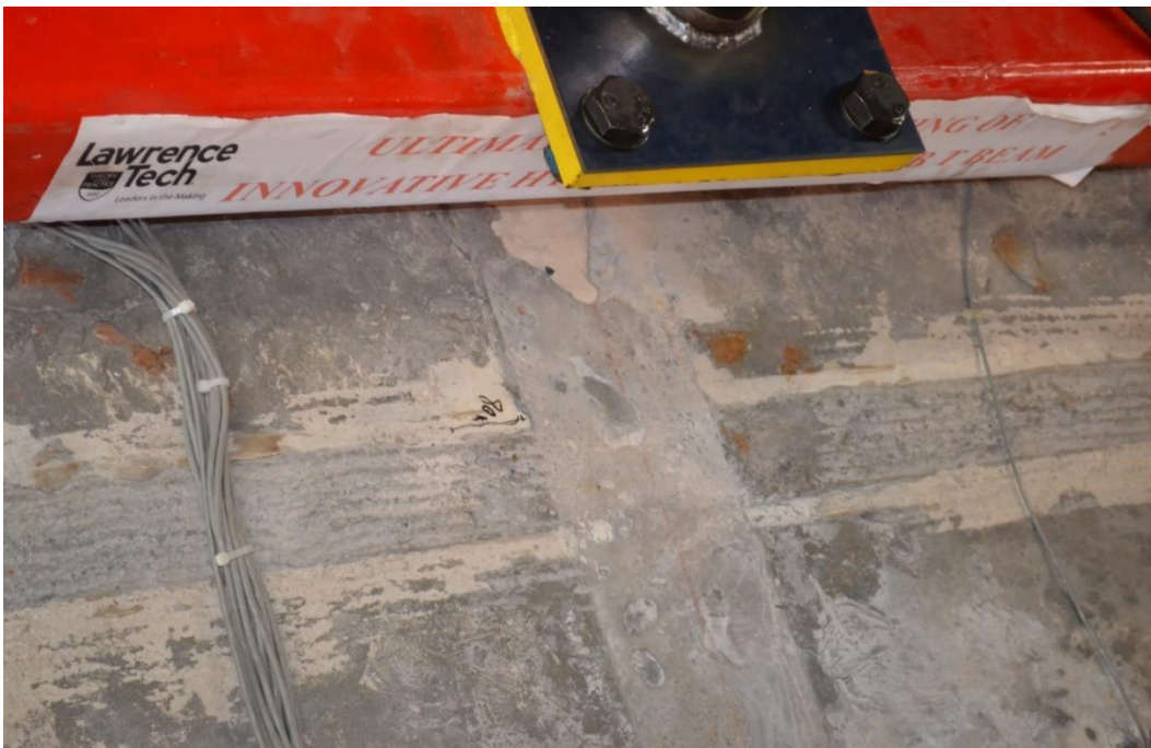
Figure 3.8-16 Localized shear key cracks at load level of 80 kip
