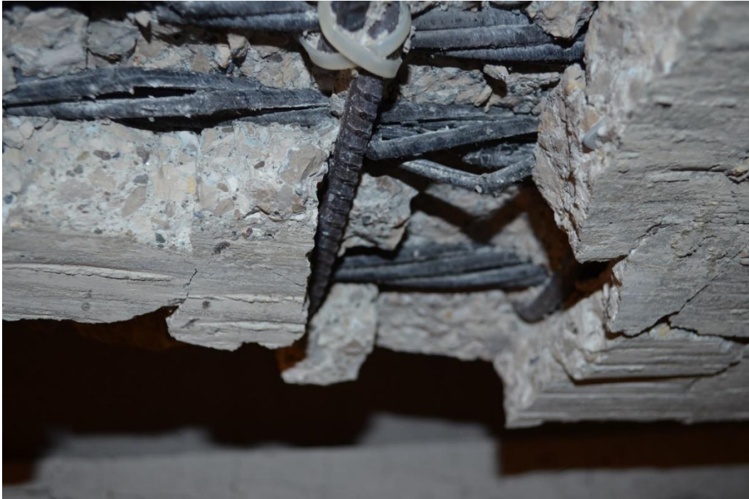
Figure 3.8-29 Rupture of prestressing CFCC strands in bridge model in intermediate beam
