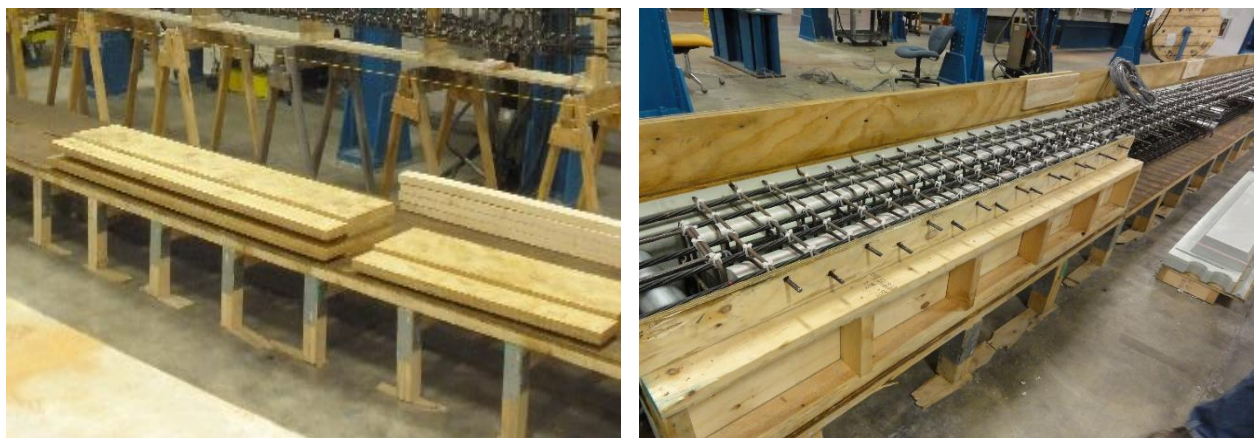
Figure 2.5-5 Sides of the formwork showing protrusion of steel stirrups for form shear key reinforcement in bridge beams
