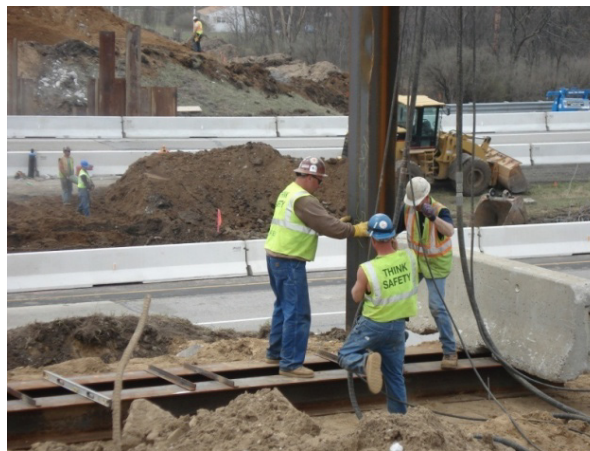
Figure 5-16. Template used for maintaining pile driving tolerances (Source: Photo courtesy of MDOT)
