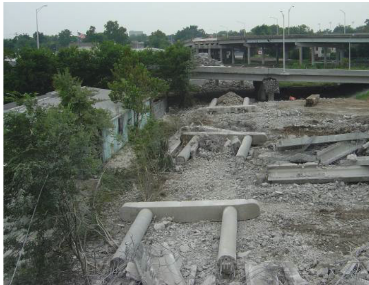
Figure 5-67. Demolition of a bent cap and columns as a single unit (Source: SCDOT)
