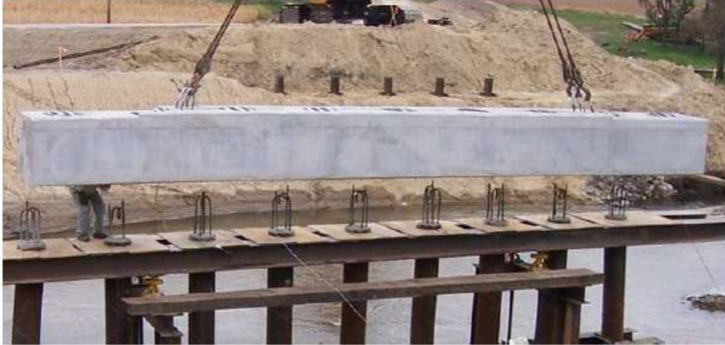
Figure 5-43. Temporary support system for pile cap to pile connection (Source: Wipf et al. 2009a)
