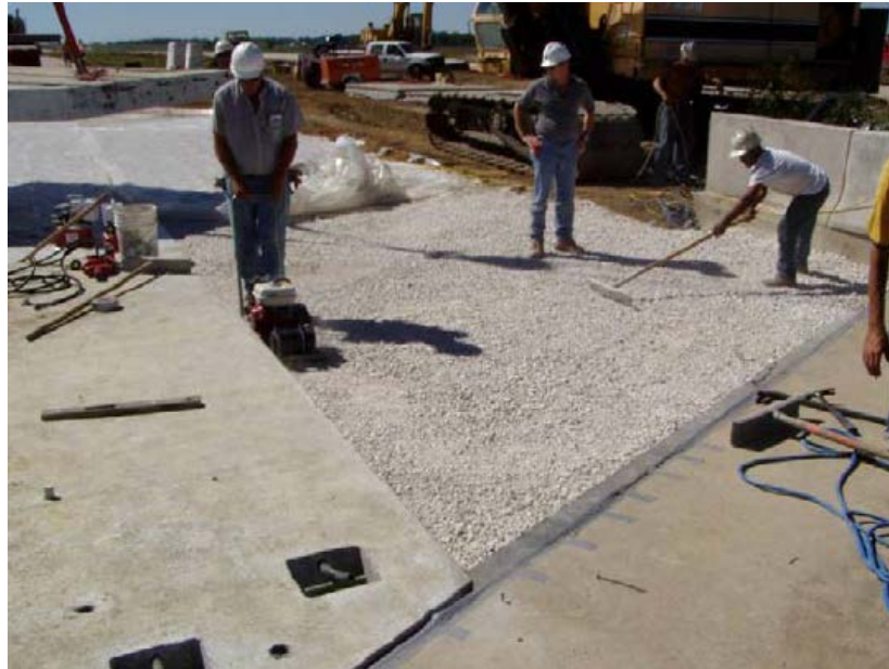
Figure 12-2 Compaction and grading of aggregate base in a PPCP BAS demonstration project in Iowa [11]
