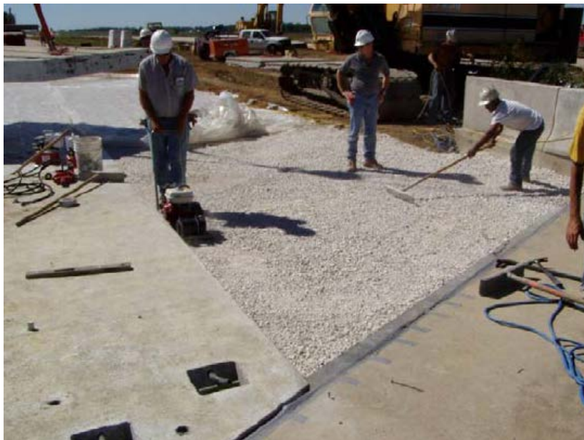
Figure 4-1 Compaction and grading of aggregate base in a PPCP BAS demonstration project in Iowa [11]
