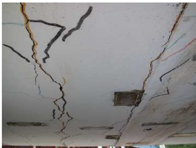
Figure 6.31: Multiple cracks under load strip
