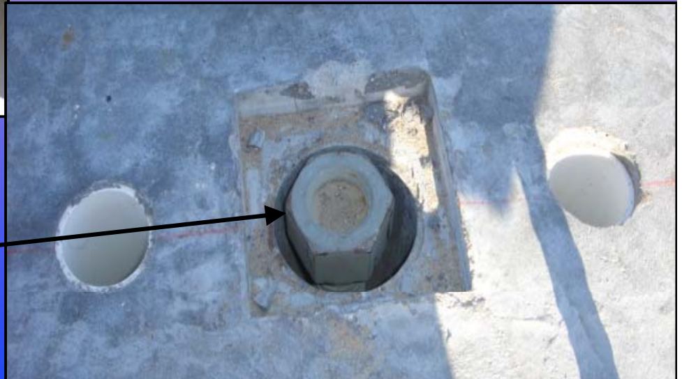
Top of Cap, Internal Support Bolt & Grout Vents
