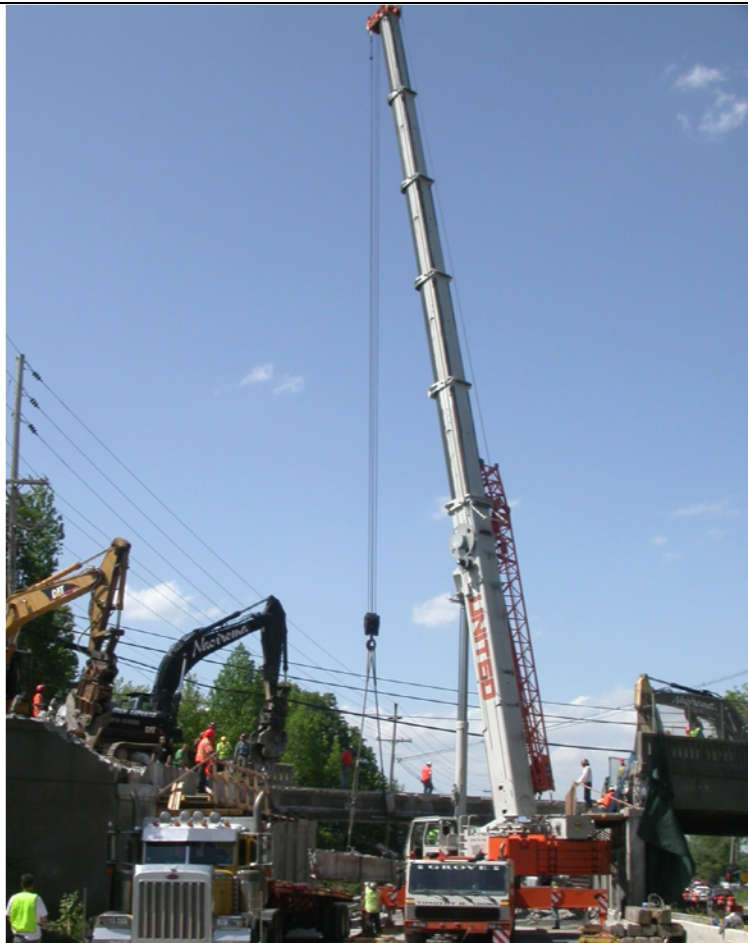
Photo 12: Crane Positioning for Beam removal, note that backwall and wingwalls are not cut (Sat 2pm).
