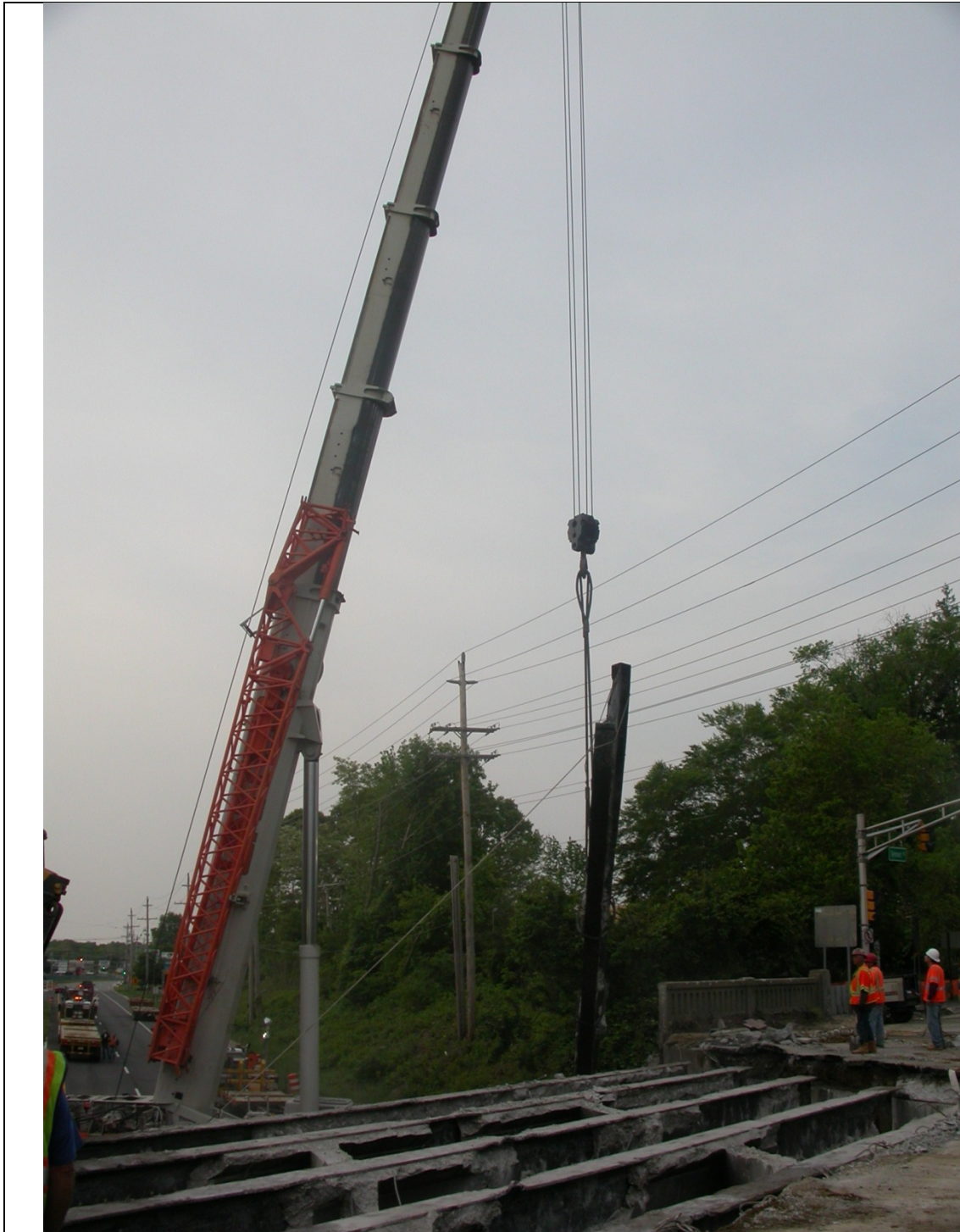
Photo 5: Continued difficulties removing Beams, note that had utilities run along the South fascia instead of the north fascia the Verizon lines could have damaged.
