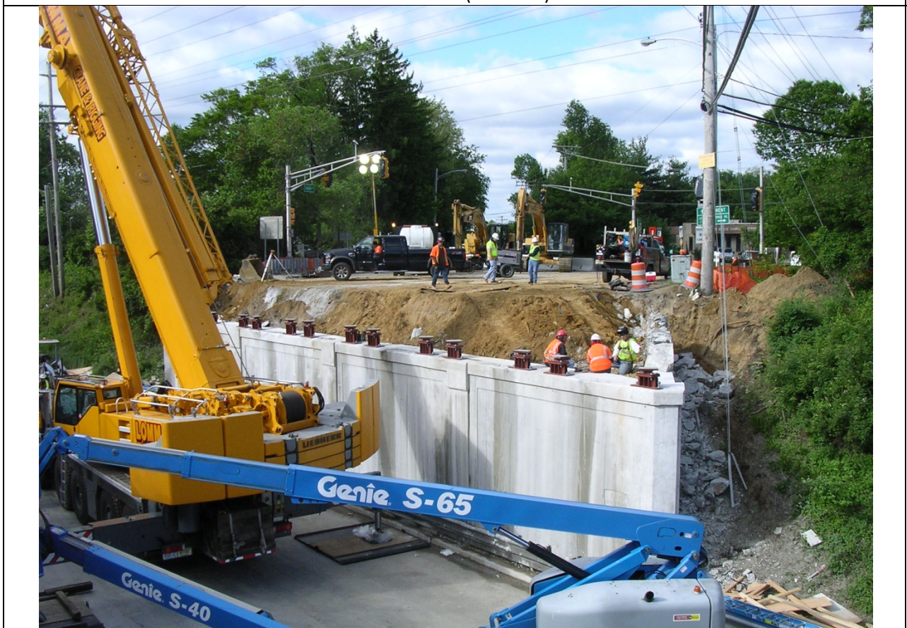
Photo 18: Bridge Seat, Bolsters, Bearings and wingwalls ready for precast sections to be placed. (Sun 8am) Note the crane shown is the 2 nd crane on the job.
