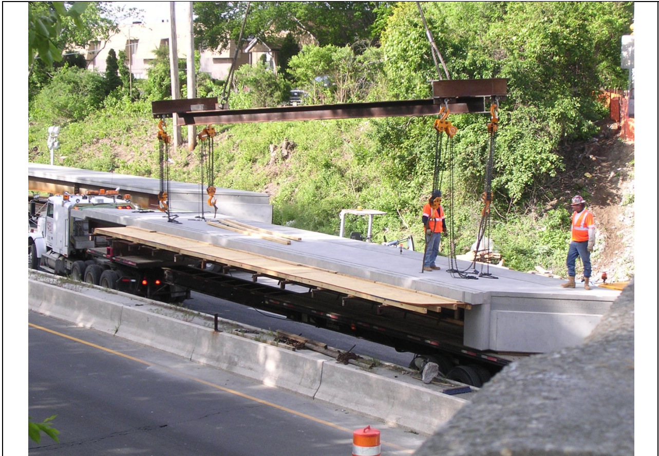
Photo 17: Attempted Use of the "Spreader Beam", which was not used due to excessive rotation of the main beam due to torsion. (Sun 8am)
