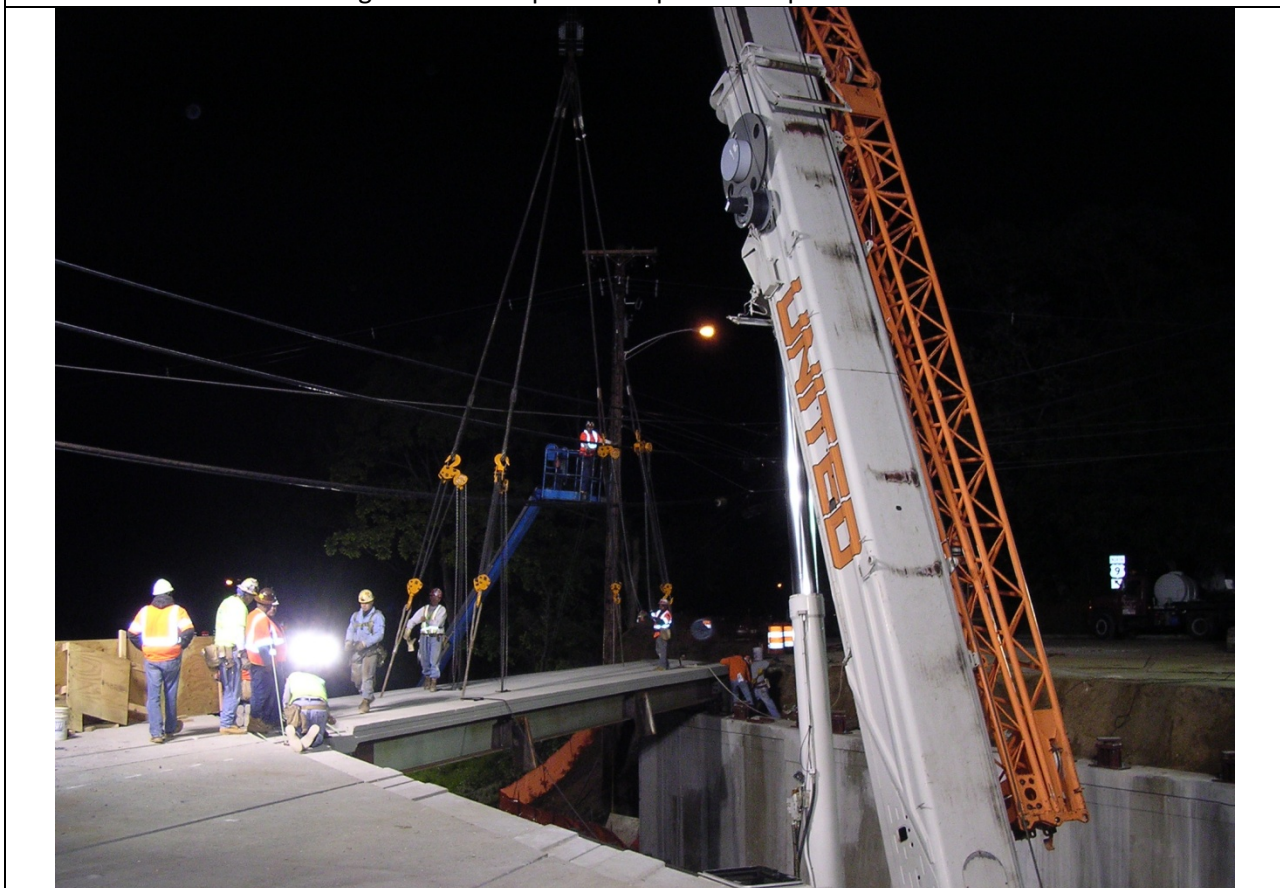
Photo 32: Weekend 2 – First precast section erected, note man in basket pulling utilities as crane sets section. (Sun 3 am)
