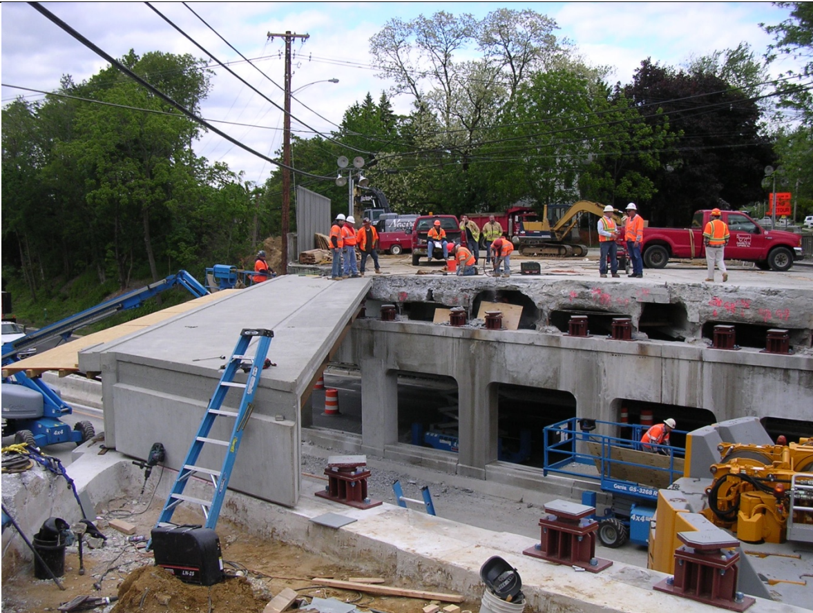
Photo 21: First Section in place. Note the orientation of the bearing with respect to the header and abutment. (Sun 4pm)
