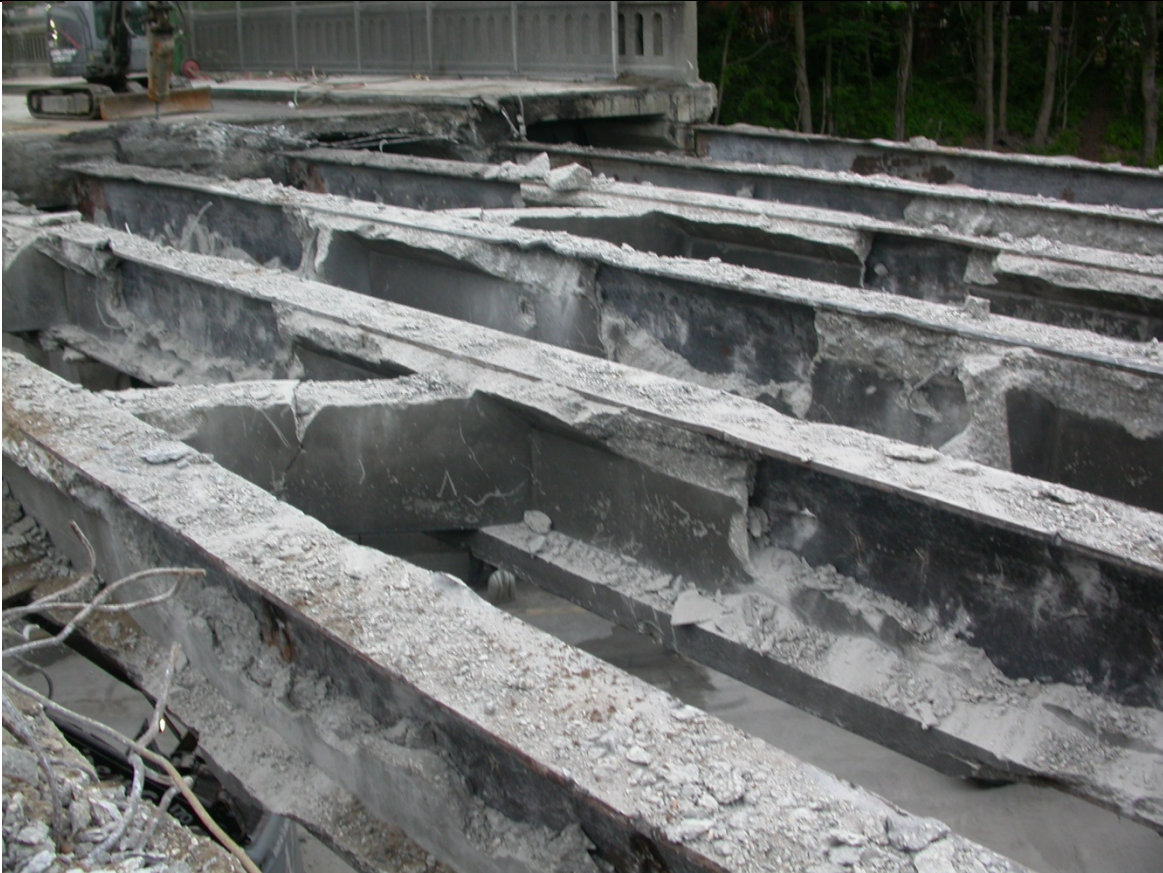
Photo 3: Extent of work to be demolished conventionally. Shown are the beams over Southbound Route 9 with deck removed – 12 hrs into Stage 3 (Weekend) Construction.
