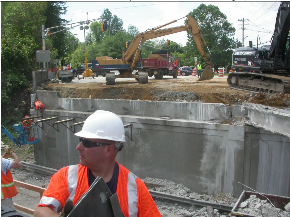
Photo 10: Backwall and Wingwalls have not been cut-down 18 hours into Demolition, the required cores for anchor bolts have not been begun.
