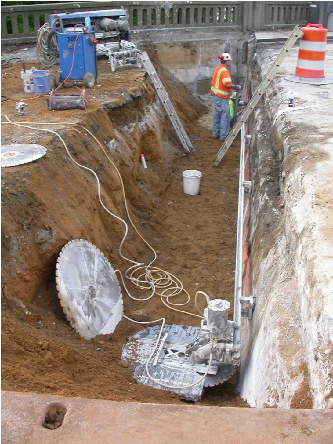
Photo 6: Extent of work cutting work remaining, backwall and wingwalls have not been removed - 12 hrs into Stage 3.
