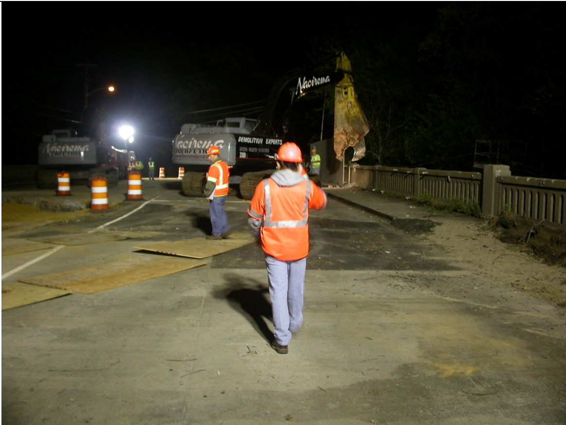
Photo 1: Balustrade removal during Stage 3 (Weekend) Construction, staging sequence suggested this to be done during Stage 2 Construction (per Sheet 31 of 56).
