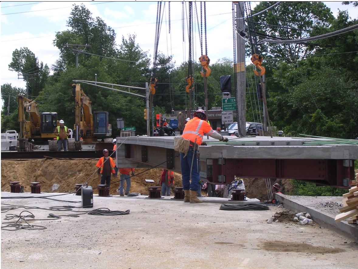
Photo 20: First Section being lifted into place. Note the number of Iron Workers/ Laborers required to land section. (Sun 1pm)
