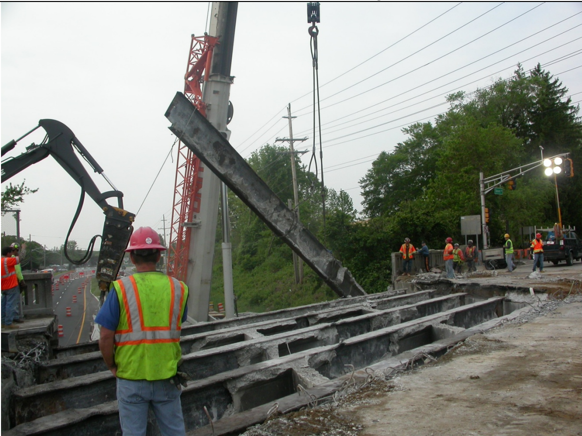
Photo 4: Difficulties removing South Fascia Beam, note that had utilities run along the South fascia instead of the north fascia the Verizon lines could have damaged.
