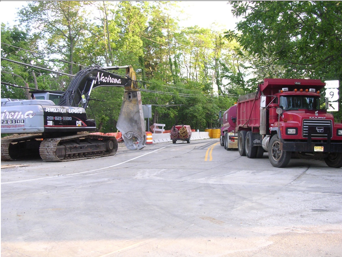
Photo 15: Staging Area at East Abutment (Contractor had proposed to use this ramp to detour Route 9 Traffic) being utilized for construction.
