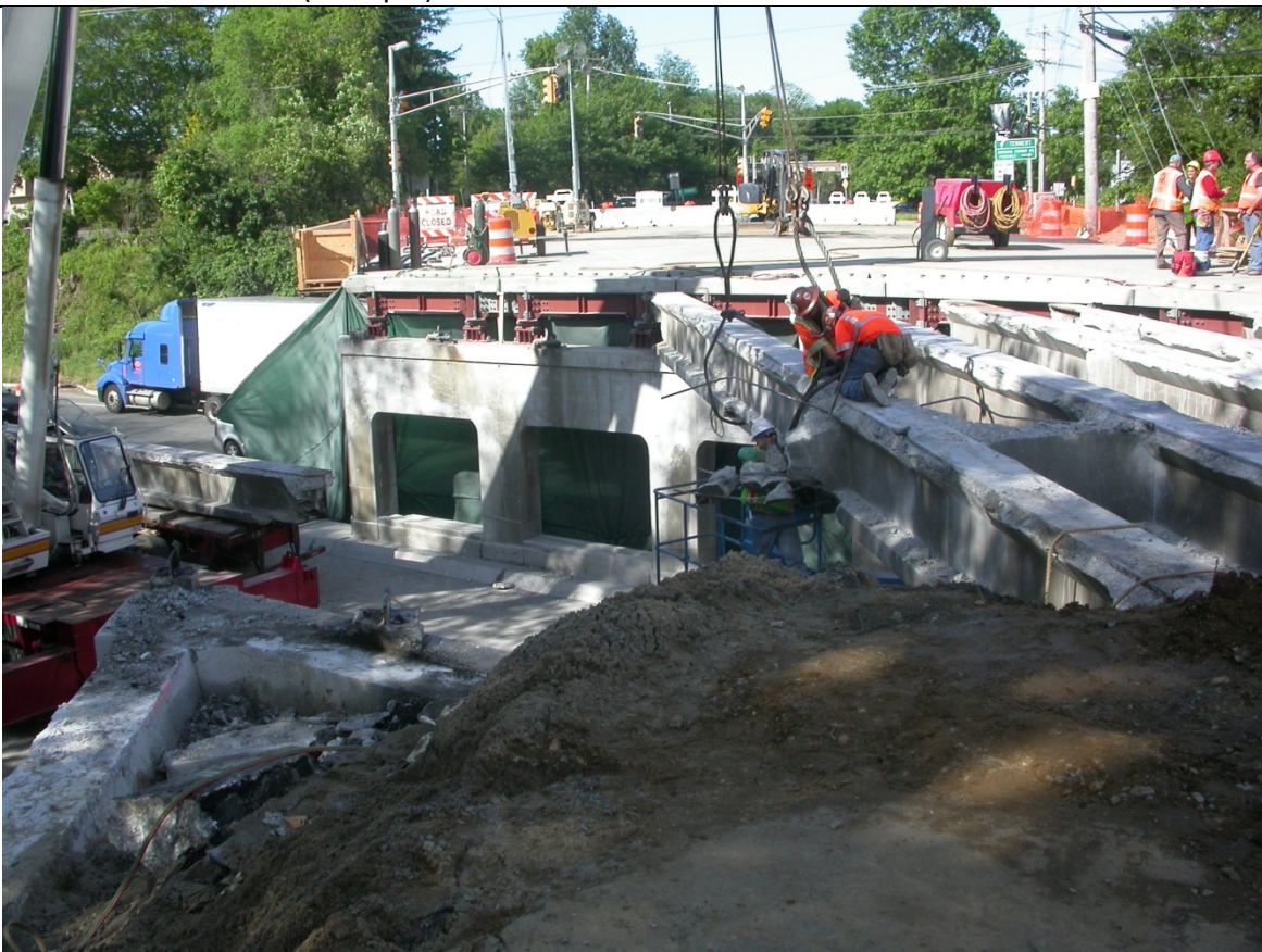
Photo 22: Weekend 2 – Three (3) Beams removed, encasement has been left on the beam during removal. (Sat 8am)
