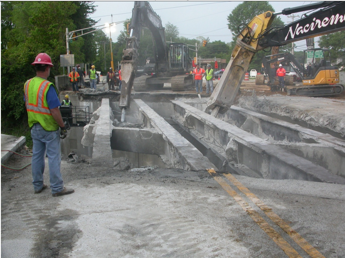
Photo 8: Contractor had to remove all diaphragms, because original demolition plan had shown that beams were to be removed in pairs, the Prime contractor had not informed the demolition contractor that they were removing beams one-by-one because the demolition technique proved inadequate.
