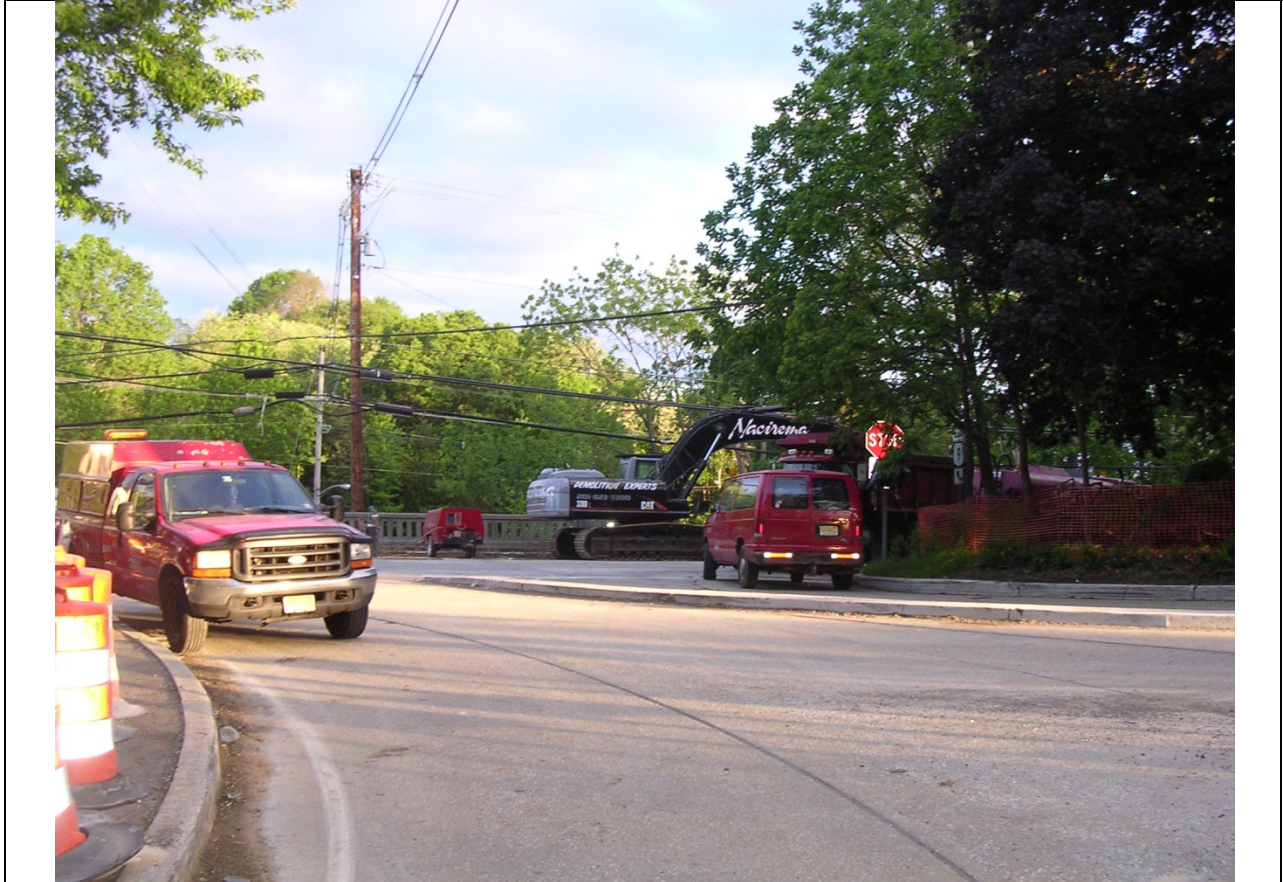
Photo 14: Staging Area at East Abutment (Contractor had proposed to use this ramp to detour Route 9 Traffic) being utilized for construction.
