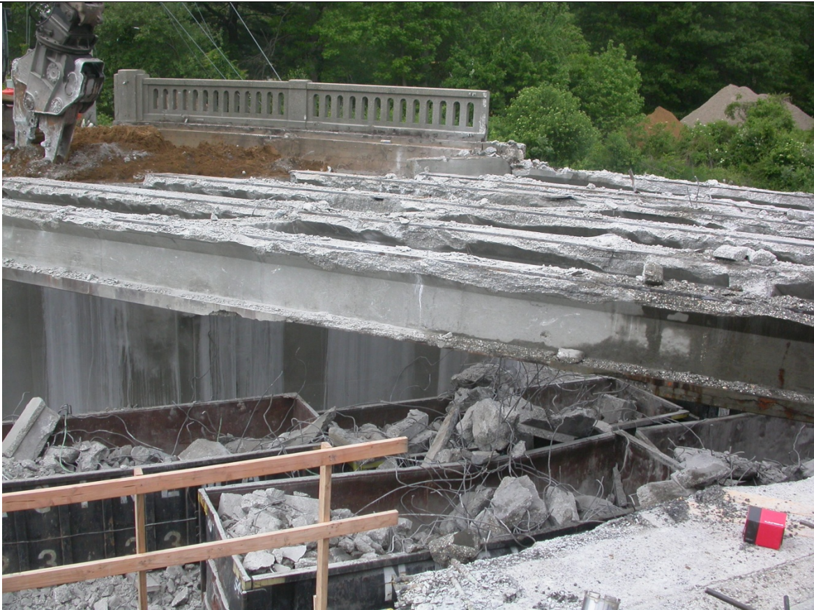
Photo 9: Dumpsters placed below the bridge to catch debris as excavators knocked deck and encasement from beams. Long periods of time were lost as dumpsters filled up and needed to be removed and new dumpsters installed. (18 hours into Stage 3)
