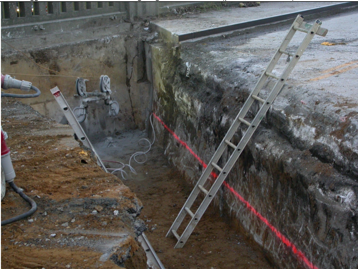
Photo 2: Backwall and South Wingwalls at Eastbound Lanes not cut during Stage 2, staging sequence suggested backwall removal and wingwall partial demo during Stage 2 (per sheet 31 of 50)
