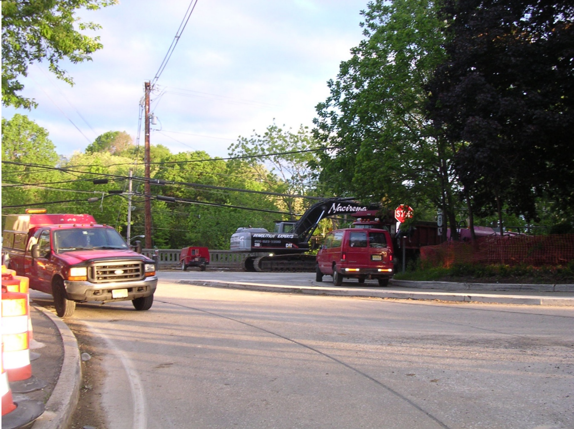
Photo 16: Staging Area at East Abutment (Contractor had proposed to use this ramp to detour Route 9 Traffic) being utilized for construction.
