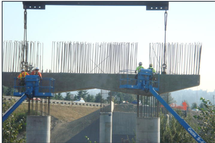
Figure 2.24 Placement of cap beam on column bars inserted in corrugated ducts in Washington State
