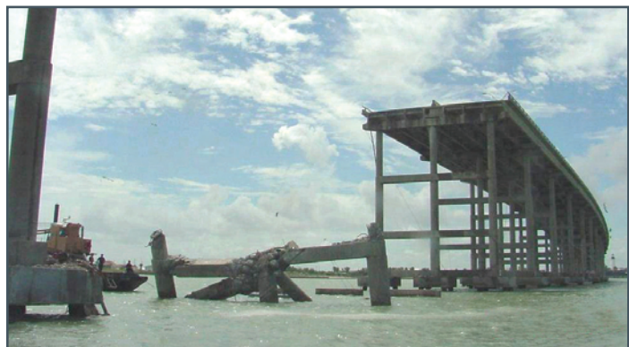
Figure 2.18 Damaged Structure after bent 31 fell on bent 32
