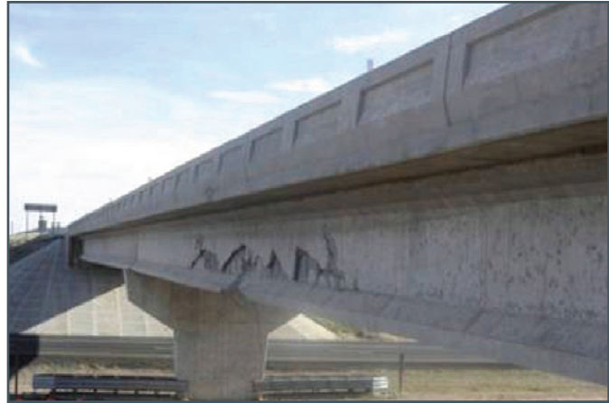
Figure 4.15 I-70 Floy interchange damaged girder
