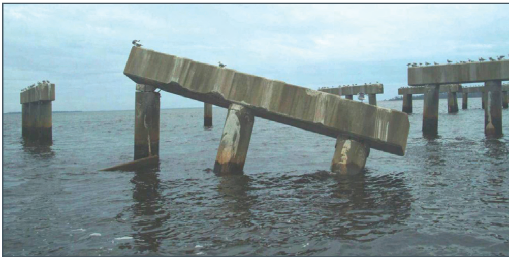
Figure 2.16 I-10 Escambia Bay Bridge's damaged piers after Hurricane Ivan
