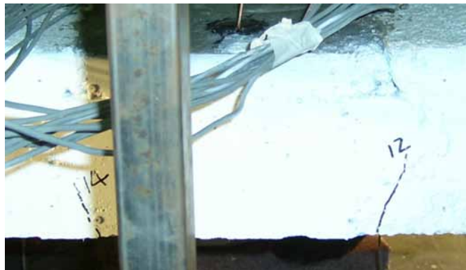
Figure 3.49. Cracks at Interface of the Joint
