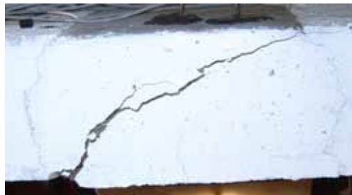
Figure 3.51. A Flexural-Shear Crack across Joint Zone
