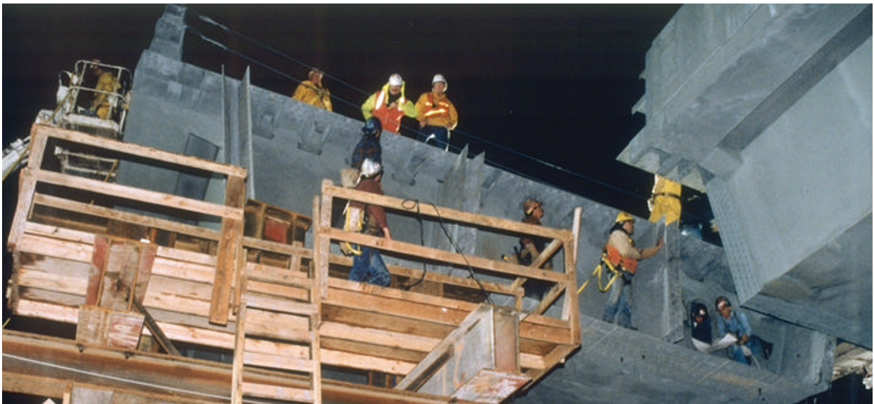
Figure 16 Ironworkers wait in position to install about 2,000 bolts to connect the second and third sections together. Before the "SHLHP" could be released some 500 of these bolts had to be torqued (A minimum of 25 percent)
