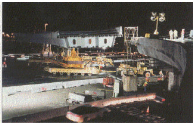
Fig. 7: Transportation of a bridge section into place (Photo courtesy of Robert Colm)
