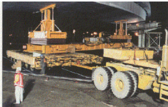
Fig. 8: Placing a bridge section into its final position (Photo courtesy of Robert Colm)
