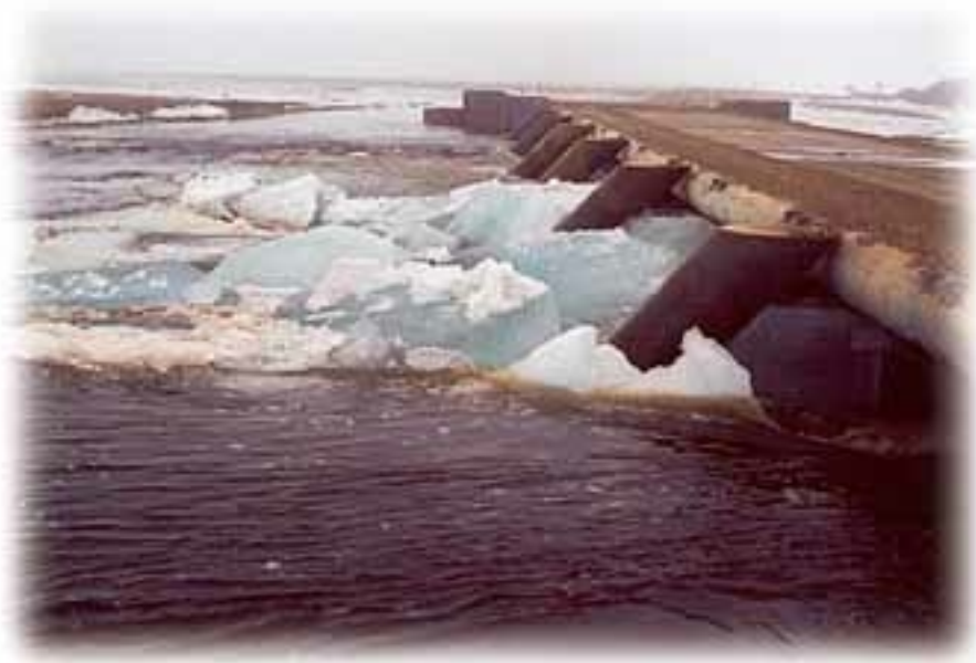
Figure 3. Five-ft (1.5 m) thick fresh water ice impacting the bridge. The thin superstructure with rounded upstream nose and the sloped ice breaking pipes were all designed to minimize the ice loading on the submersible bridge, and to provide ice passage over or under the bridge.
