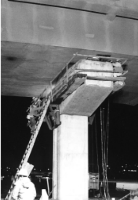
Figure 5. Two welders each field-weld a top bearing plate to connect the bottom of the section to the previously installed bearing.
