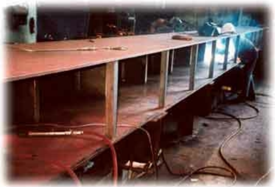
Figure 2. Fabrication of the pile cap. Angle braces were welded to the base of the webs to minimize distortion/warpage and to support the bottom flange during fabrication.
