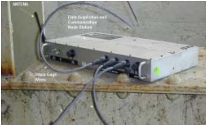
Figure 2.1 - Wireless Structural Monitoring System with Node Station Hard-wired to the Strain Gages but Wireless to the Base Receiver through Antenna
