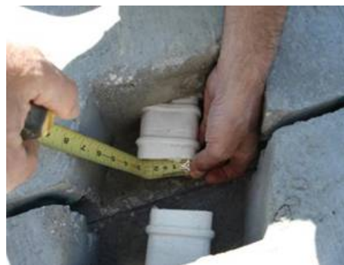
1(b) Post-tension duct misalignment
