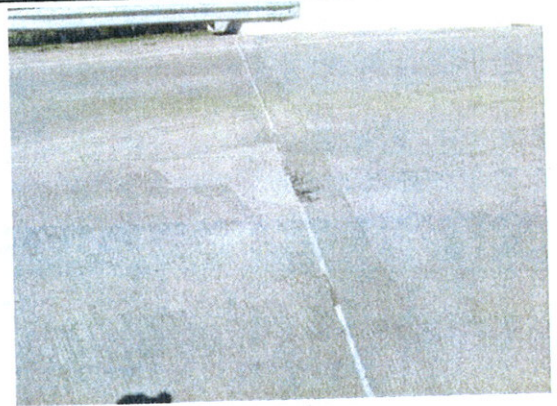
PATCH ON APPROACH SLAB AT SOUTH END
