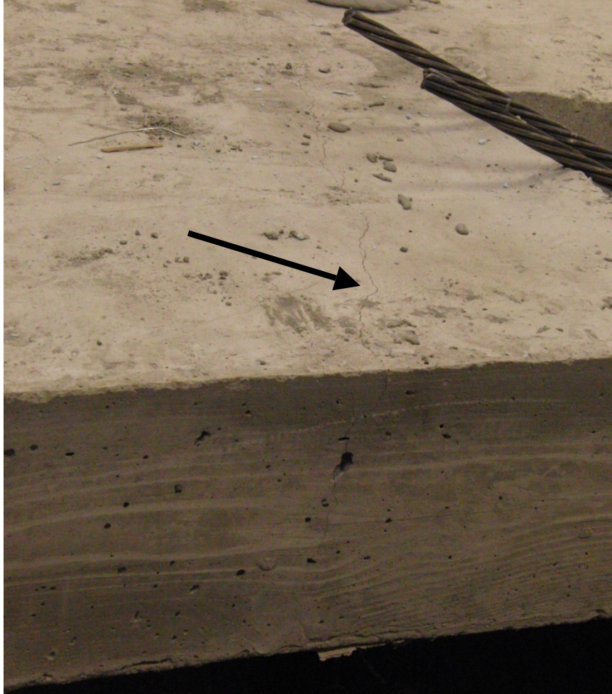
Figure 32: Flexural Cracking of Deck Panel Away from Joint.
