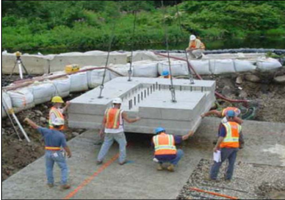
Figure 65. Precast Concrete Footing Being Lowered into Position on Native Subgrade. Mill Street Bridge over Lamprey River, New Hampshire. (FHWA 2009.)
