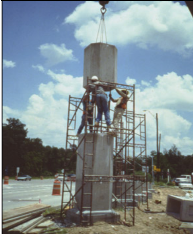
Figure 18. Assembly of Precast Segmental Columns on Louetta Road Overpass. (CABA, ND Slide 24.)
