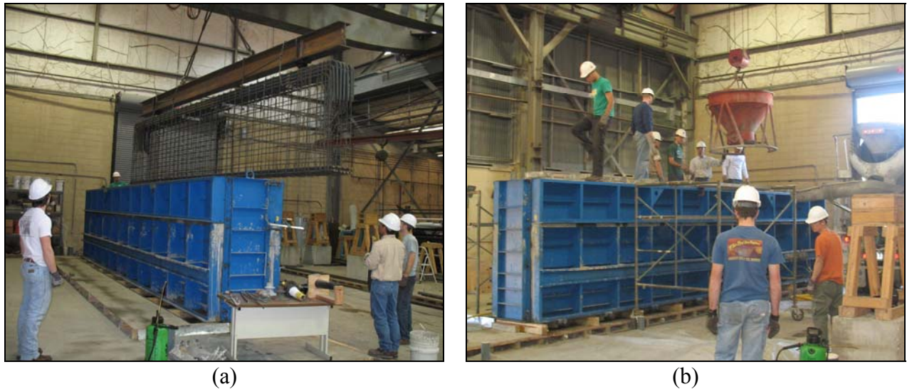
Figure 3.21: Fabrication of a 21''x75'' beam: (a) movement of reinforcement cage into formwork (b) placement of concrete into steel formwork
