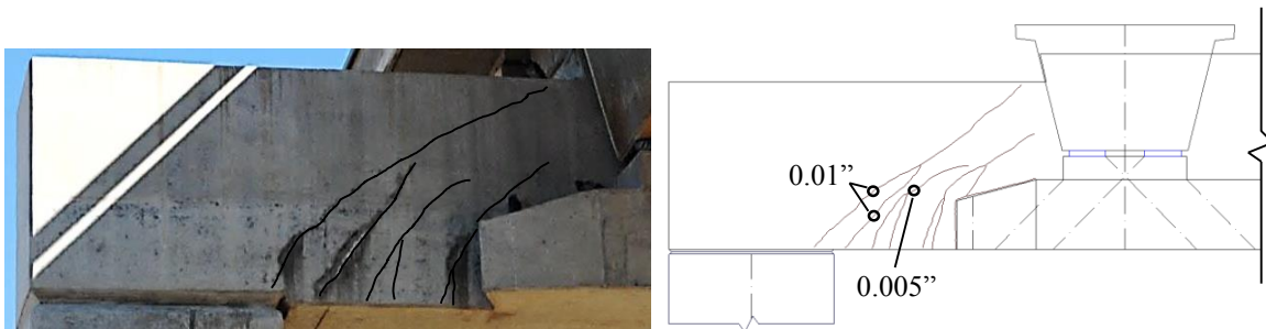
Figure 6-24: Crack Size and Location on the Southwest Corner of Waco Bent 17
