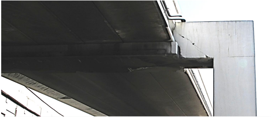
Figure 2-1: Severely distressed inverted-T bent cap in El Paso.
