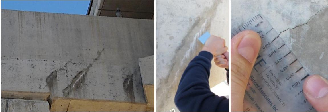
Figure 6-23: Scraping off Efflorescence and Measuring Diagonal Cracks
