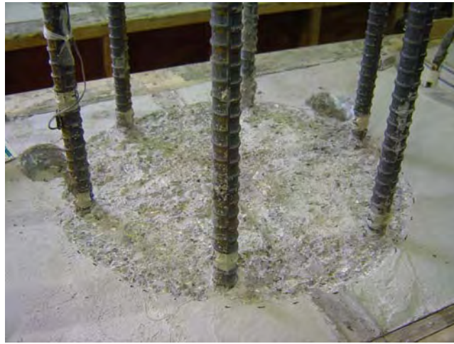
Figure B-32: Roughened surface of cap-beam under grout pad
