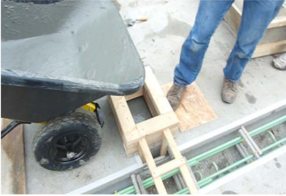
a) Pouring UHPC joint fill into shear pocket using a wheel barrow
