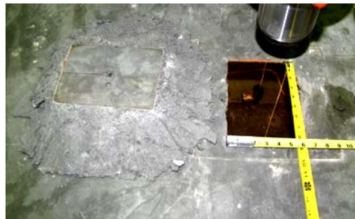
c) Punching failure surface
