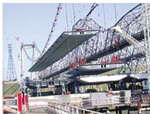
UNIQUE Combo of strand jacks, trestles and skids set orthotropic deck sections. (Photo courtesy of FCI)
