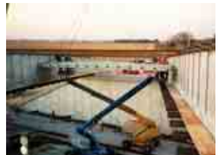
Deck panels sit against shear keys at the bottom of the girders. After post-tensioning, grout will be used to close the gap between the edges of the panels and the girders.
