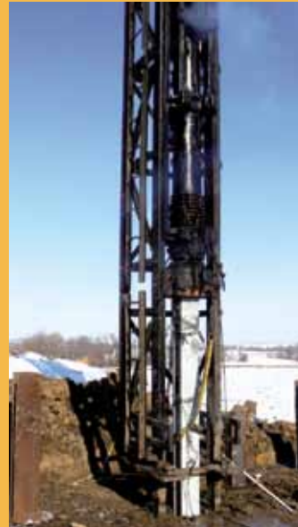
A UHPC pile driven at the test site: drivability characteristics were evaluated and the pile load tested
