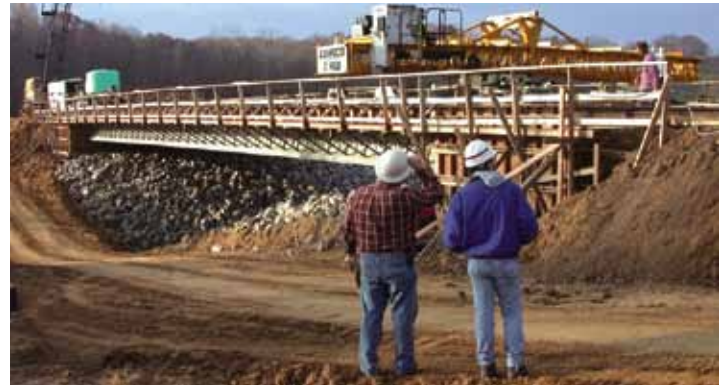
Figure 1 – The first UHPC bridge built in the United States is located in Wapello County, Iowa.
