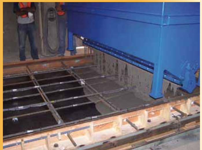
UHPC placement of test panel form at Coreslab Structures Inc., Omaha, Neb.
