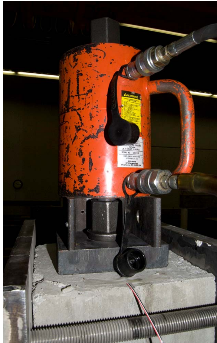
Figure 4: Post-Tensioning Jack and Anchorage
