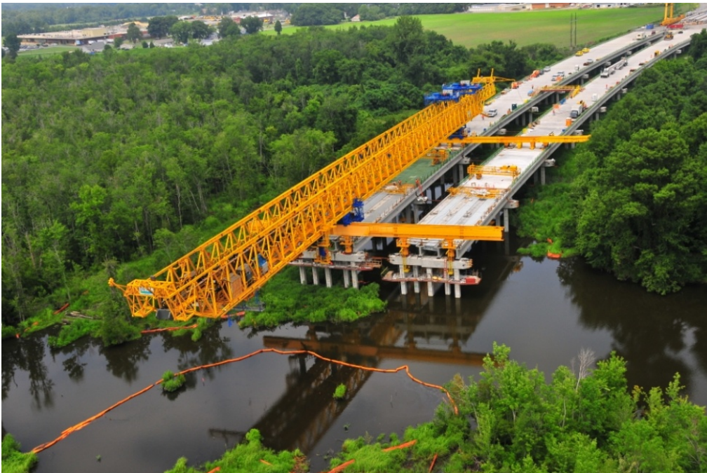
Fig. 8: Launching Gantry 2 over Kennedy Creek, with Minimal Impact of the Pile Driving to Wetlands Below
