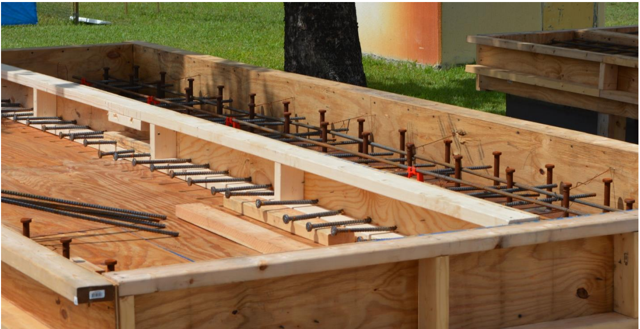
Fig. 5. Showing construction of the headed bar closure pour detail, modeled after Bridge A.
