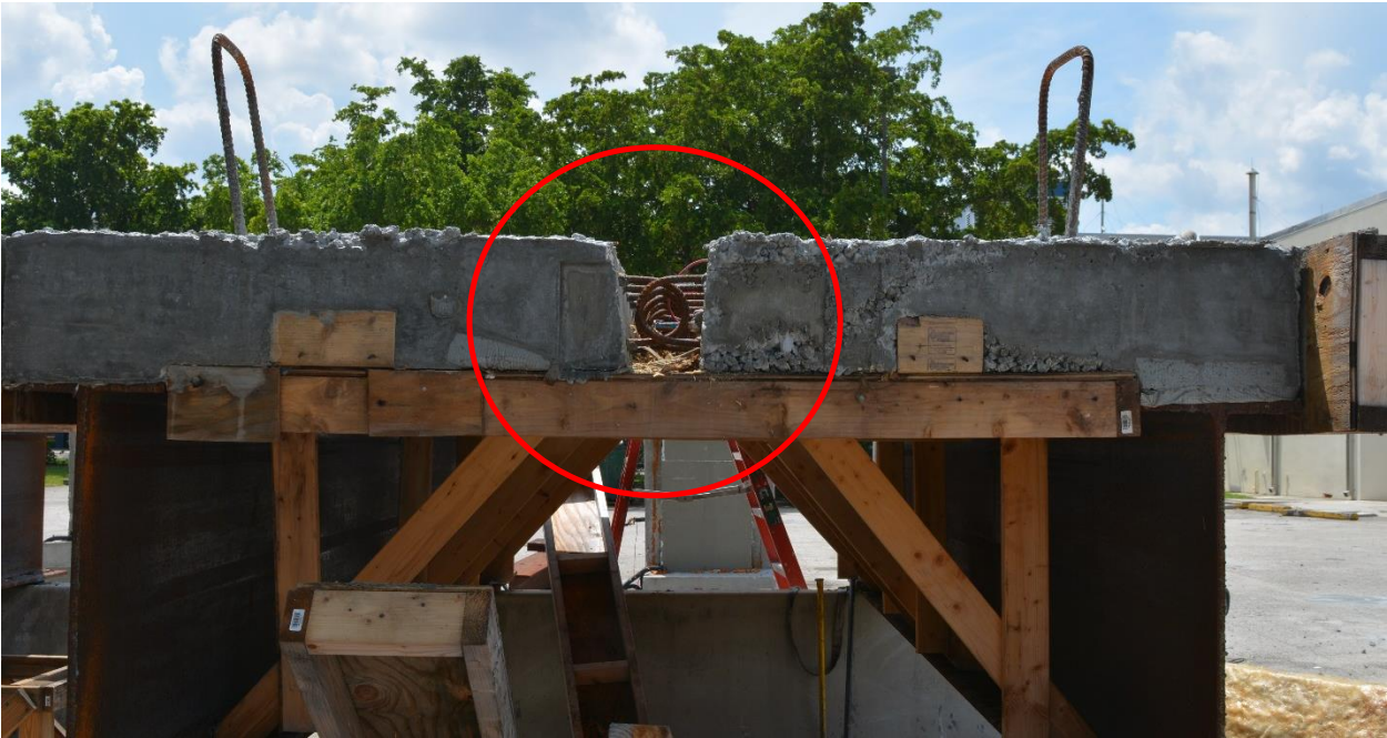
Fig. 9. Hairpin detail, note lack of keyway on this end.
