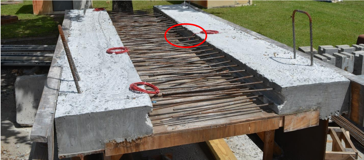
Fig. 8. Mass 14 detail, note bars are not extending through joint.
