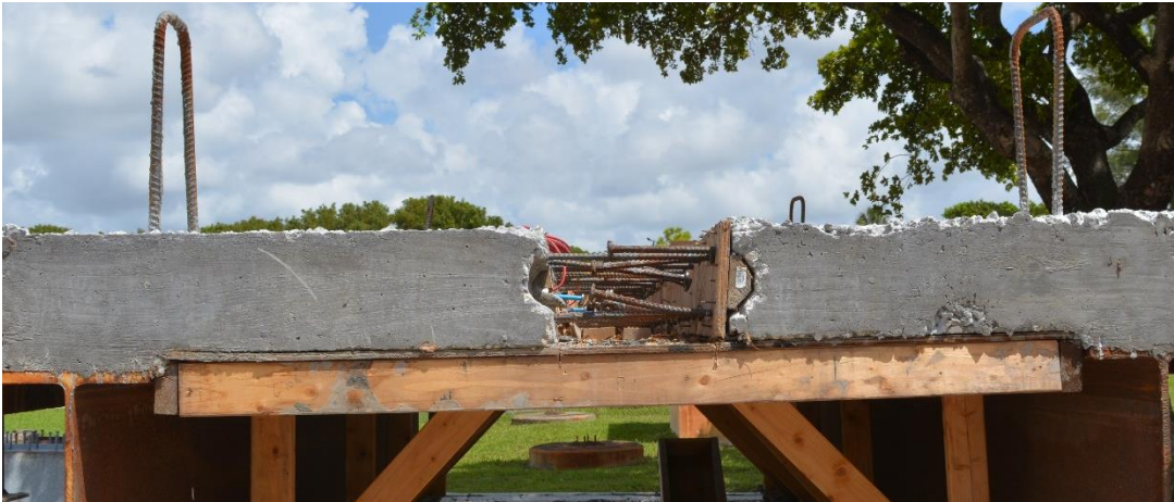
Fig 7. Showing headed bar detail. Note that forms have not been completely removed.
