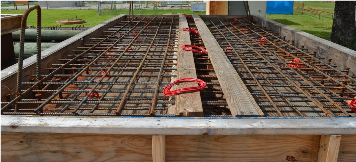
Fig. 6. Showing construction of the closure pour detail with hairpin bars, modeled after Bridge B.
