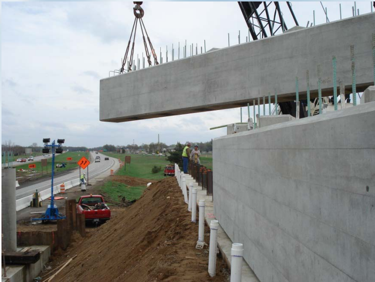
Photo Credits: Michigan DOT
