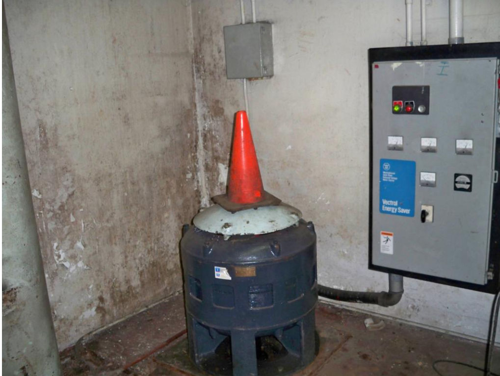
Photo 3: motor and electrical panels
