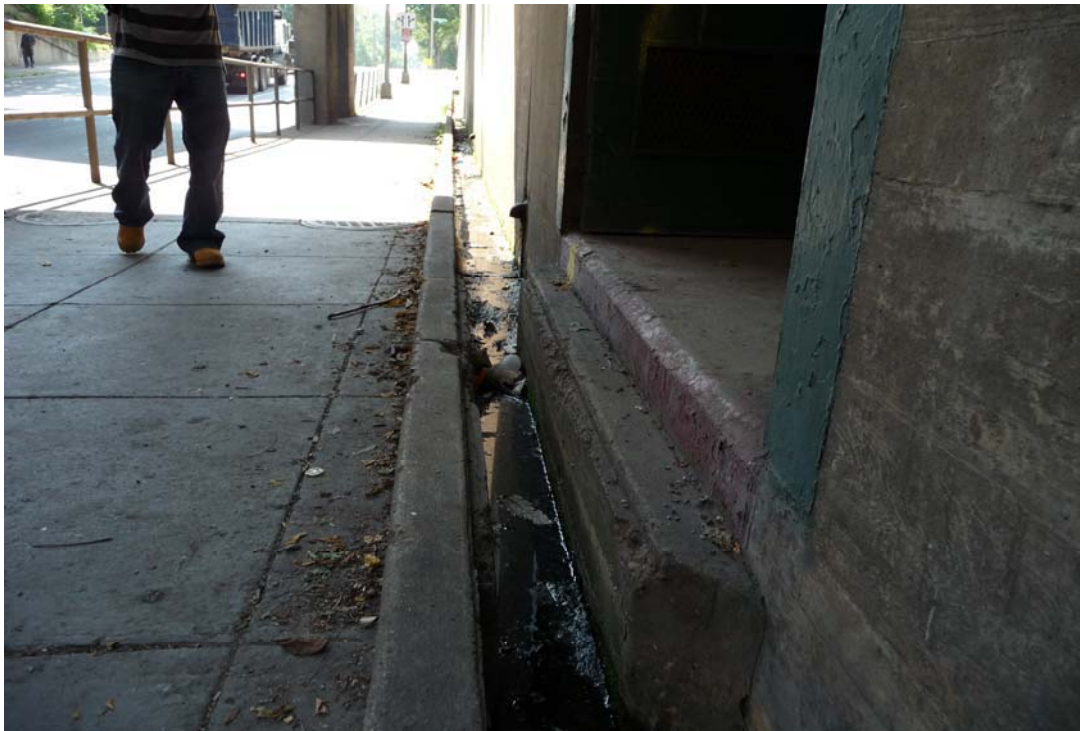
Photo No. 2- Drainage Ditch at Front Door
