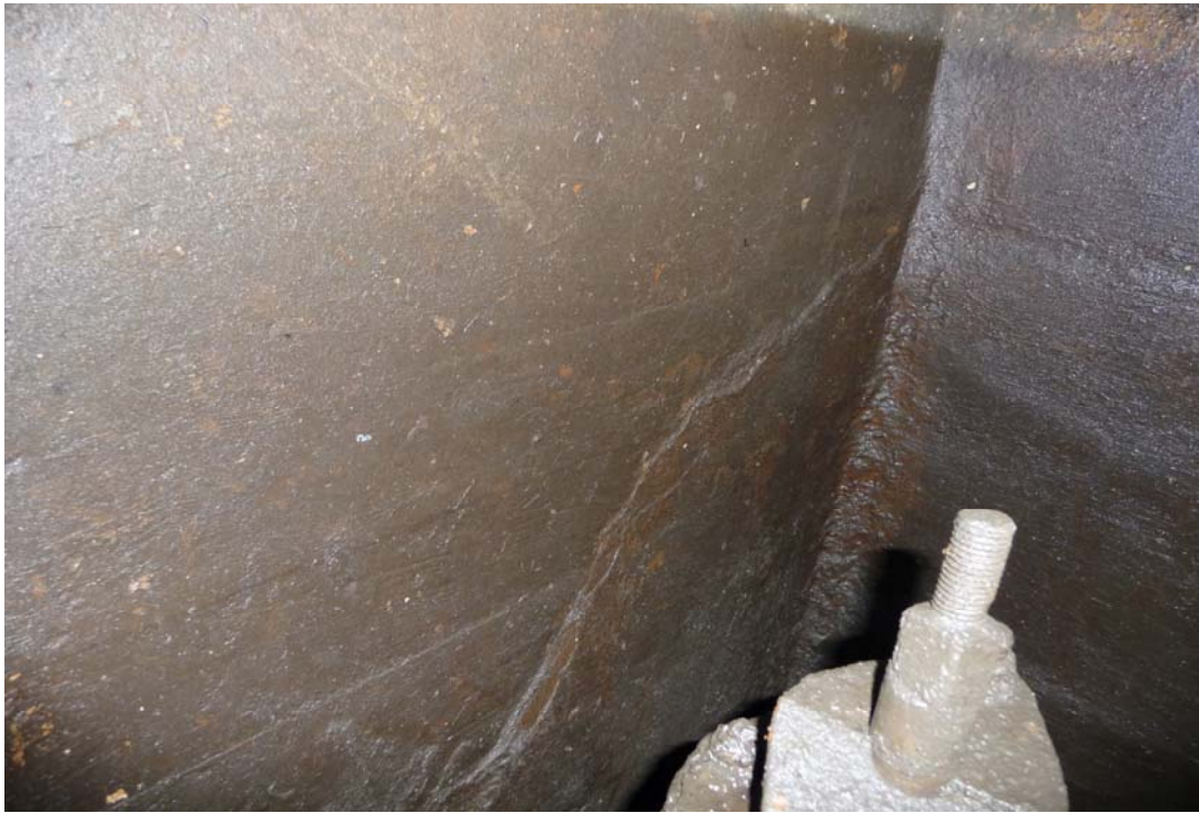
Photo No. 9- Pump Chamber, Crack on Wall
