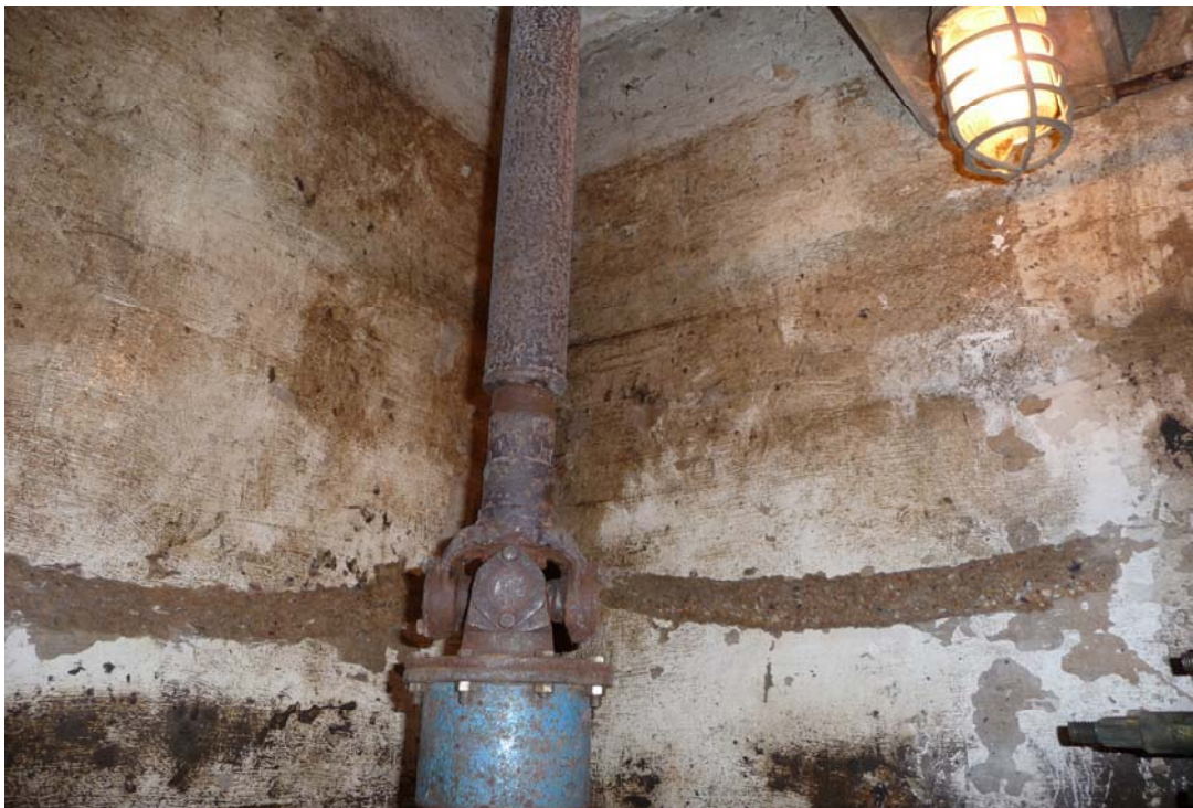
Photo No. 12- Pump Chamber Walls, Concrete Spall
