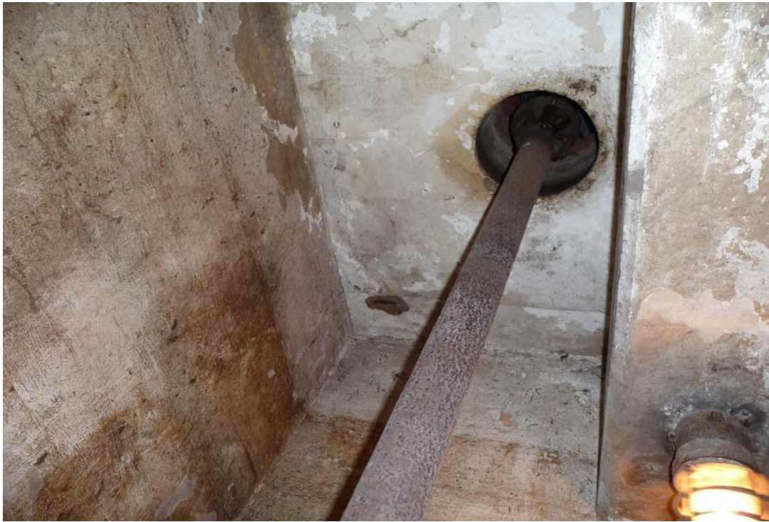
Photo No. 11- Pump Chamber, Spall and Exposed Rebar on Ceiling
