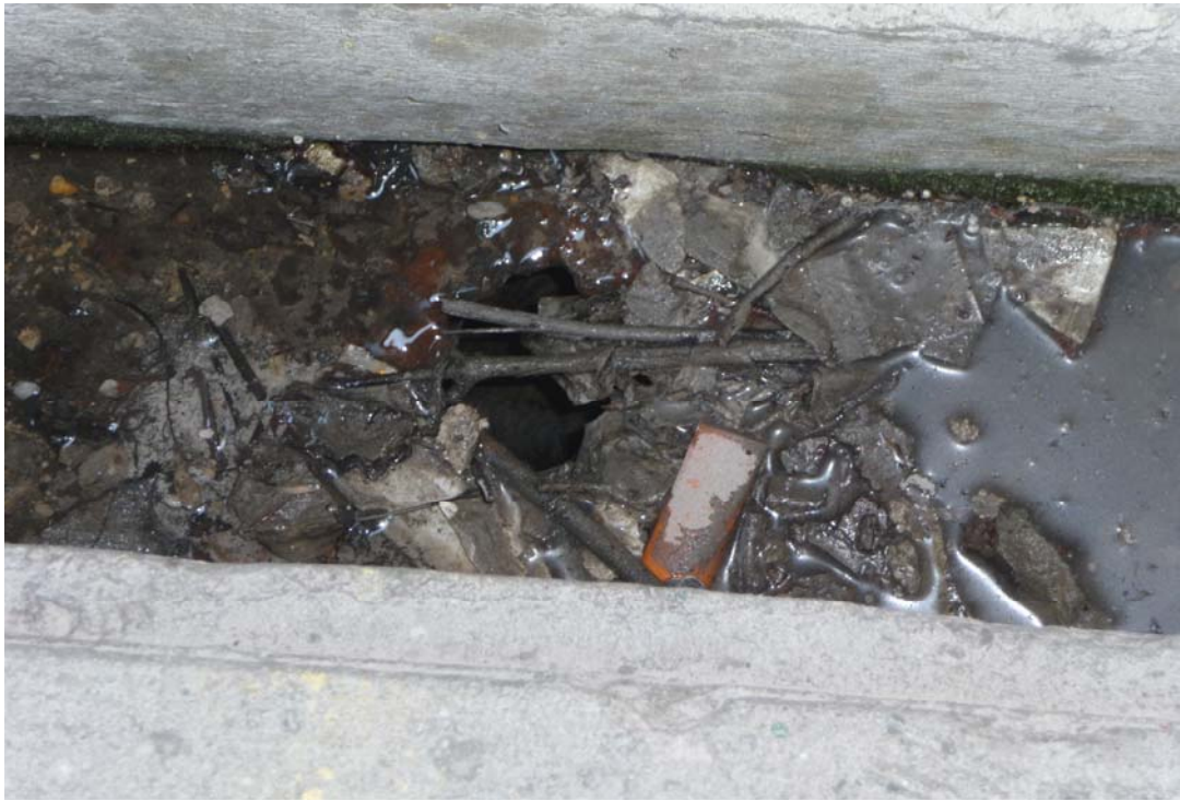
Photo No. 3- 3" Hole at Bottom Slab of Drainage Ditch
