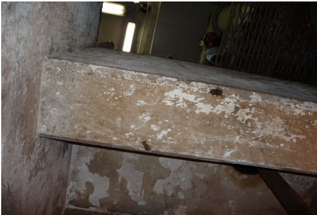
Photo No. 10- Pump Chamber Ceiling, Spall and Exposed Rebar under the Beam
