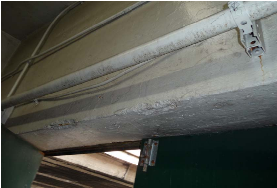
Photo No. 7- Motor Room, Wall at top of Door Opening
