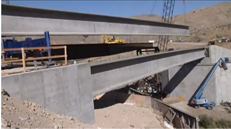
Figure 33. Second girder transferred from the girder launcher to the bent abutments during construction of the superstructure.
