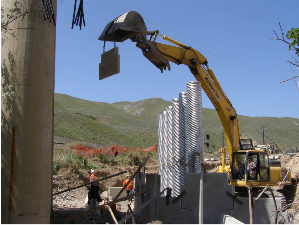
Figure 25. Installing MSE retaining wall around the corrugated metal pile spacers (side view).
