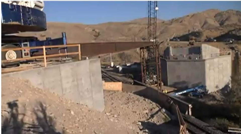
Figure 30. Completed installation of falsework to temporarily support the girders during construction of the superstructure.
