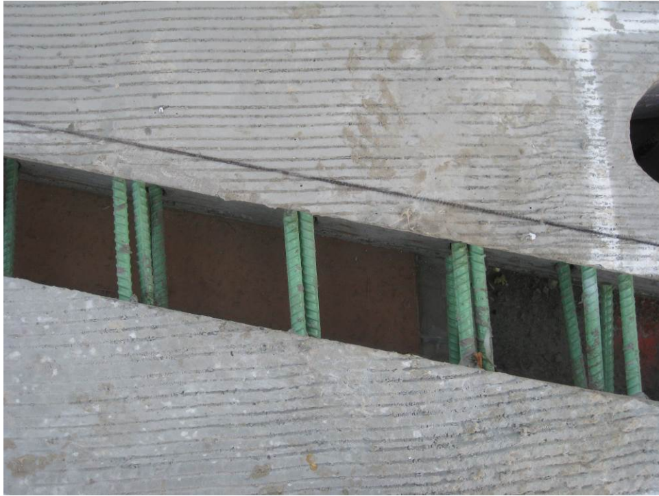
Figure 45. Close-up of the joint between the deck panels. Below the joint is the top of the girder and the wooden forms to hold the UHPC in the transverse joints.
