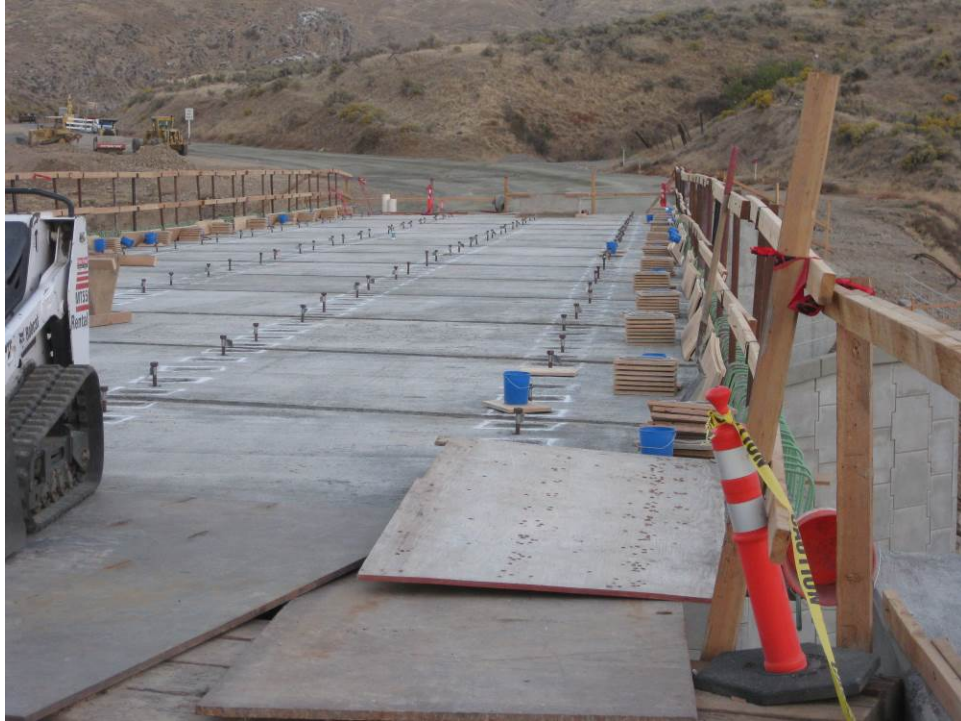
Figure 37. View of the deck from south end of the bridge following installation of all prefabricated bridge deck panels.
