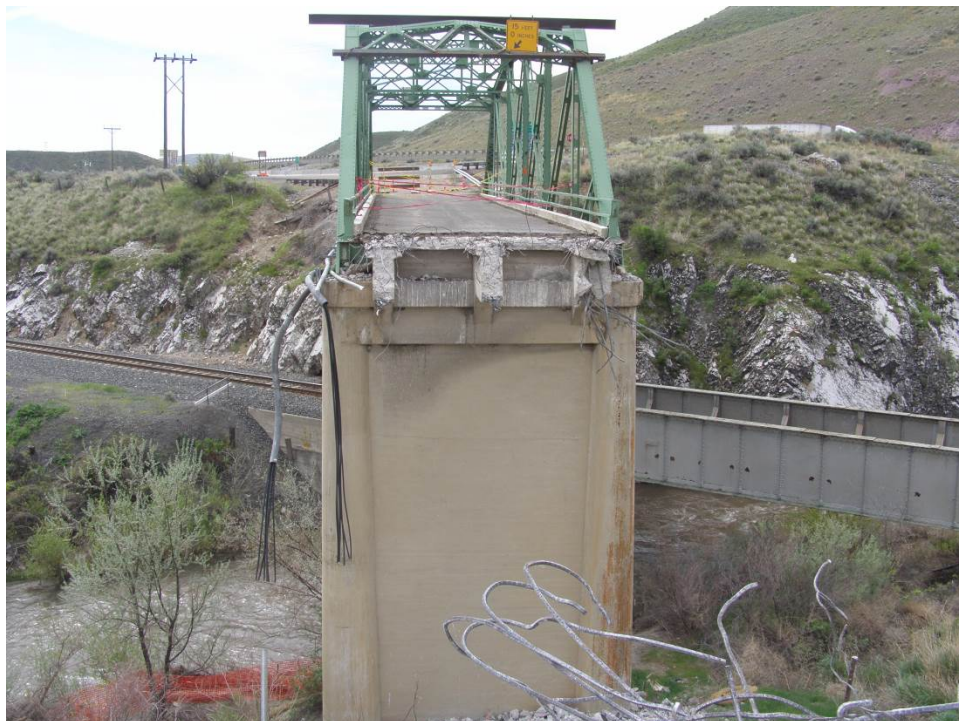
Figure 18. Demolished approach of brige 0700.
