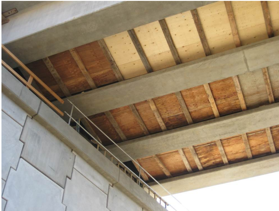
Figure 46. View of the reinforced concrete girders and the wooden forms to hold the UHPC in the transverse joints from underneath the bridge deck.
