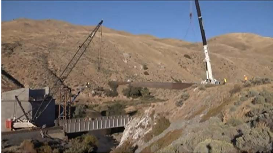
Figure 29. Installation of falsework to support the girders during construction of the superstructure.
