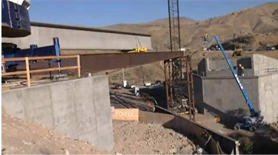
Figure 31. Girder being rolled onto the temporary support during construction of the superstructure.
