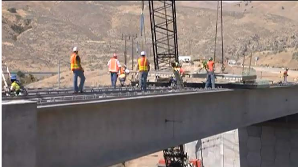
Figure 35. Installation of the second prefabricated bridge deck panel (P9) during construction of the superstructure.
