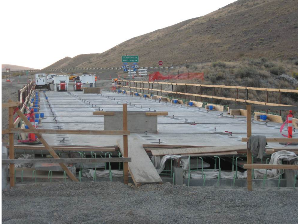
Figure 39. View of the deck from north end of the bridge following installation of all prefabricated bridge deck panels.
