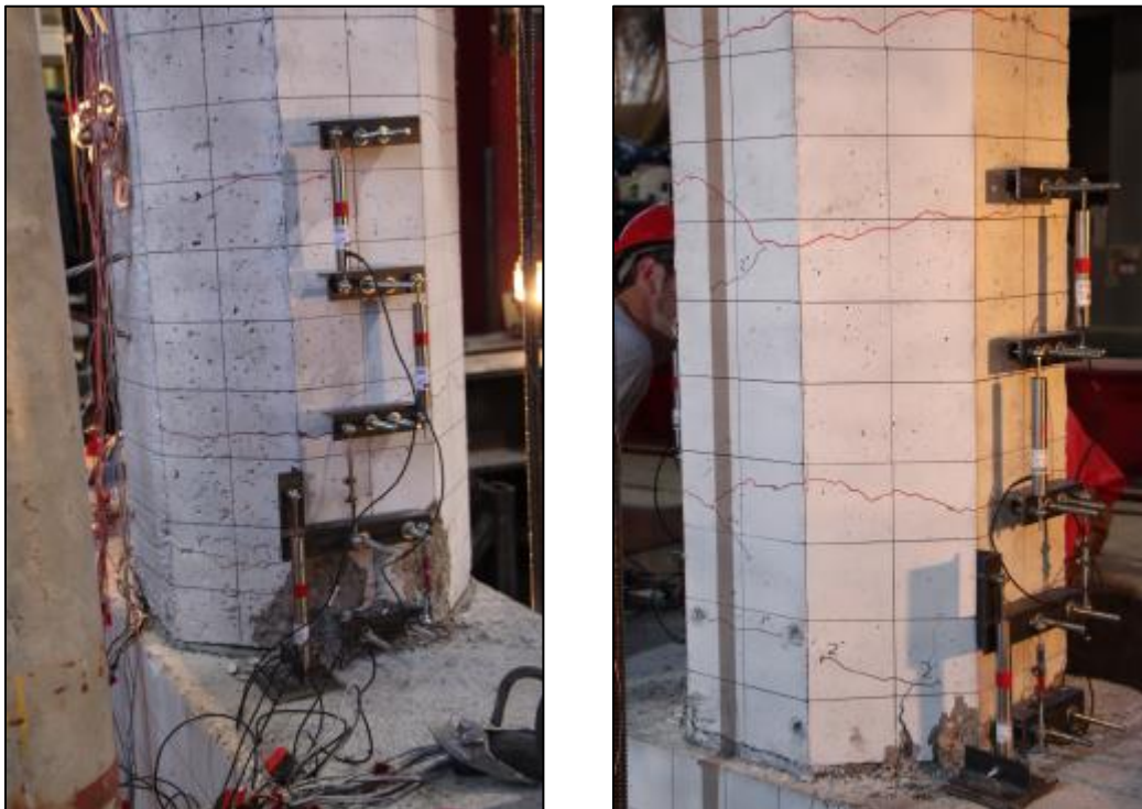
Figure 4-46. Damage state for FGSS-3 at 4% drift ratio.
