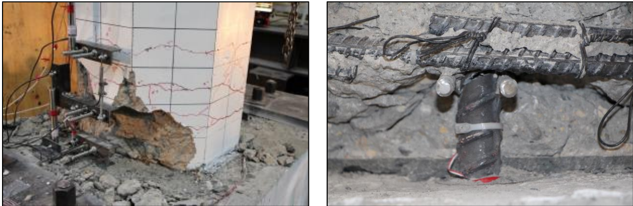
(b) Damage state at 7% drift ratio: cracks, spalling, fractured bar, and exposed rebar cage.
