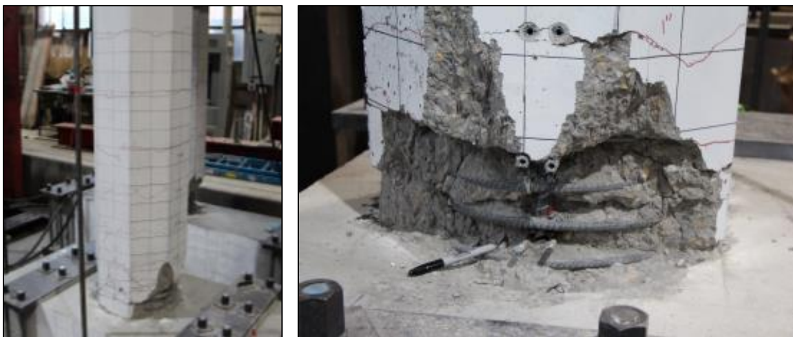
(c) Damage state at end of test: cracks, spalling, concrete delamination, and fractured rebar.
