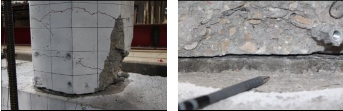
Figure 4-48. Damage state for FGSS-3 at end of test: cracks and spalling, permanent gap.
