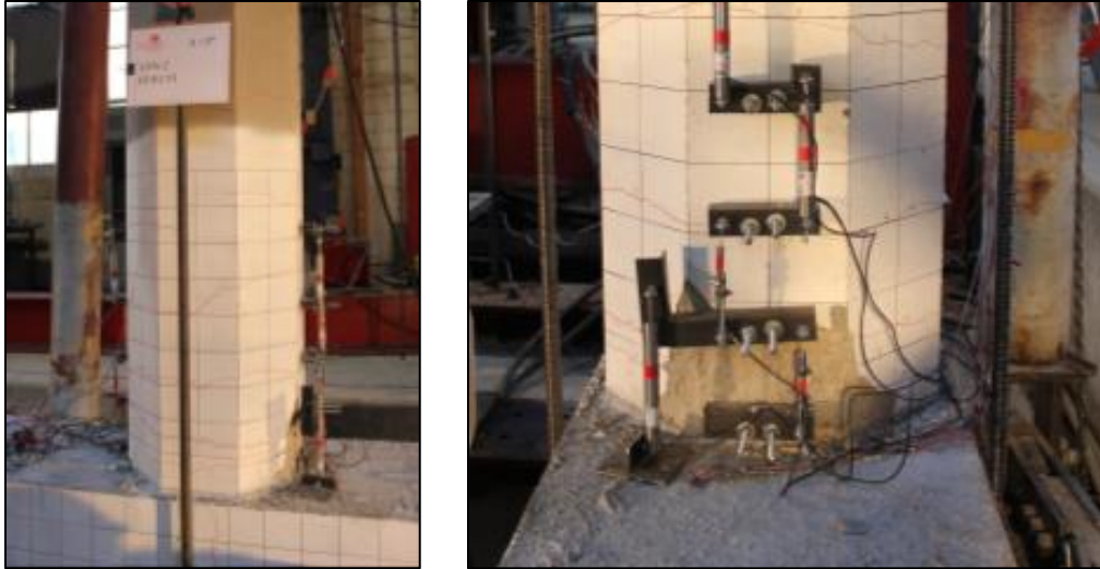
(a) Damage state at 3% drift ratio: cracks and spalling.
