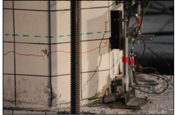
(b) Damage state at 3% drift ratio.
