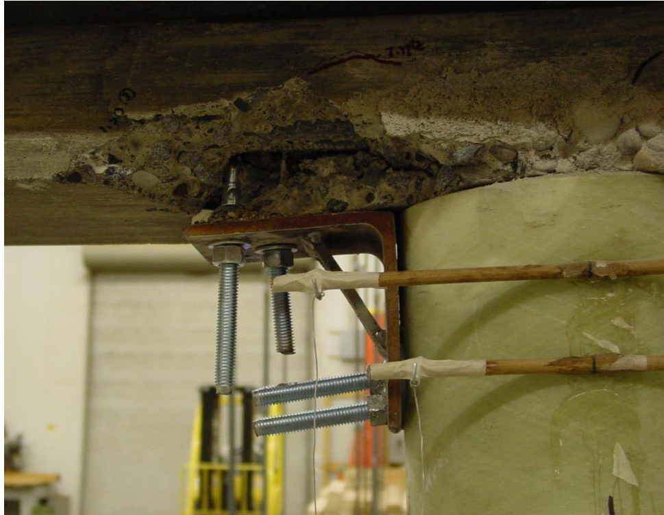
Figure 5.2.29: Pull-out of concrete surrounding the bolts fixing the northern modified steel angle to the beam at the 3.40 in. displacement cycle
