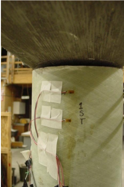
(a) Gap at column-beam interface of northern column
