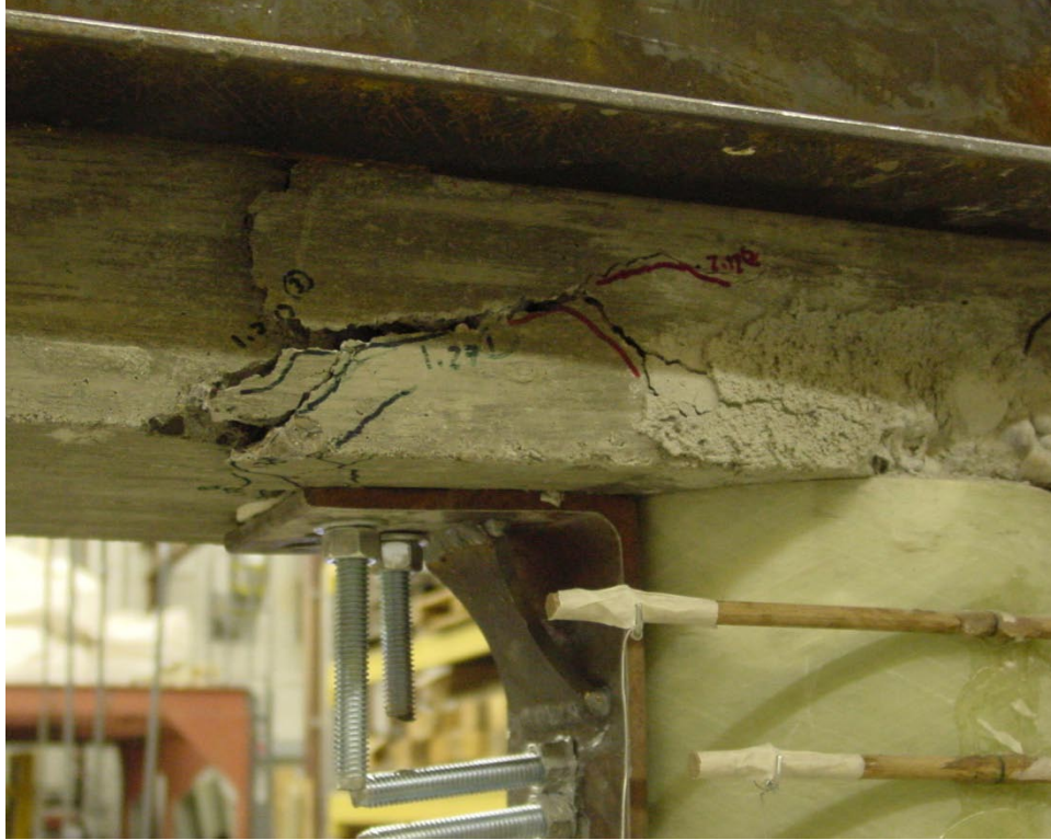
Figure 5.2.28: Concrete began to spall at the northern corner of the beam of specimen F-FRP3-S after the 3 rd cycle of the 2.12 in. displacement level
