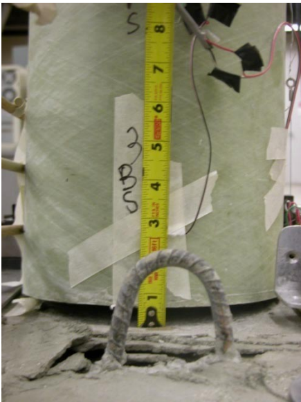
(c) Gap at column-base interface of northern column
