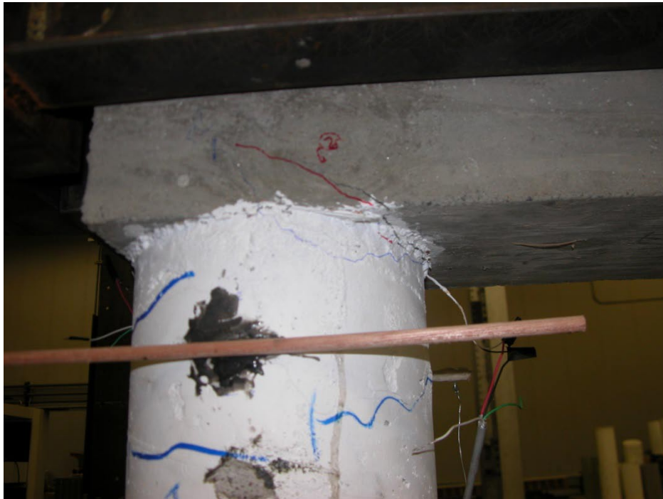
Figure 5.2.4: Cracks extending to the beam at 1.40 in displacement
