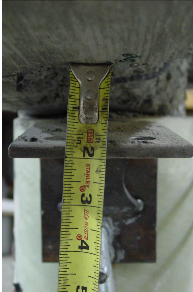
Figure 5.2.34: Gap opening between steel angle and beam bottom surface at the north corner of the beam during maximum displacement
