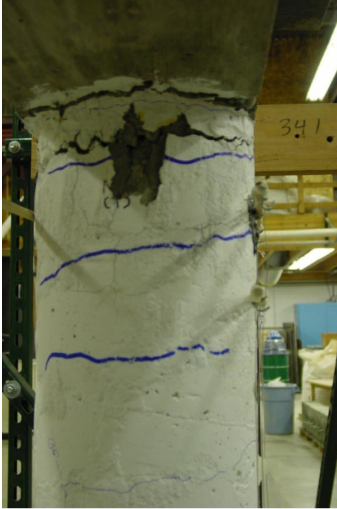
Figure 5.2.5: Concrete spalling at 2.7 in. displacement
