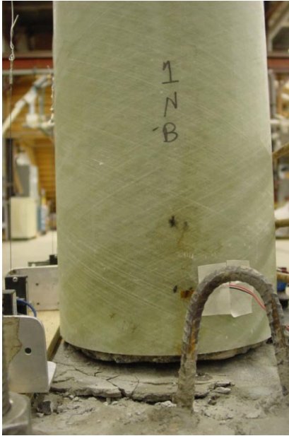
(c) Gap at column-base interface of northern column
