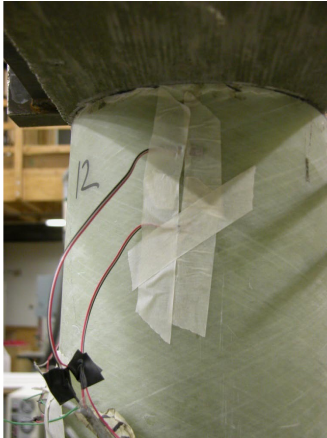
Figure 5.2.20 (b): Damage to FRP tube of specimen F-FRP3 at column beam-interface of northern column
